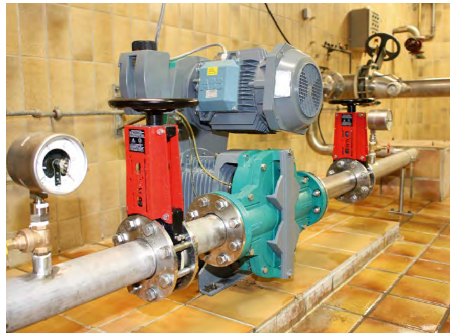
Centrifuge feed: 2 % DS excess sludge at a flowrate of 18 m 3 /h against a discharge pressure of 1,5 bar.
