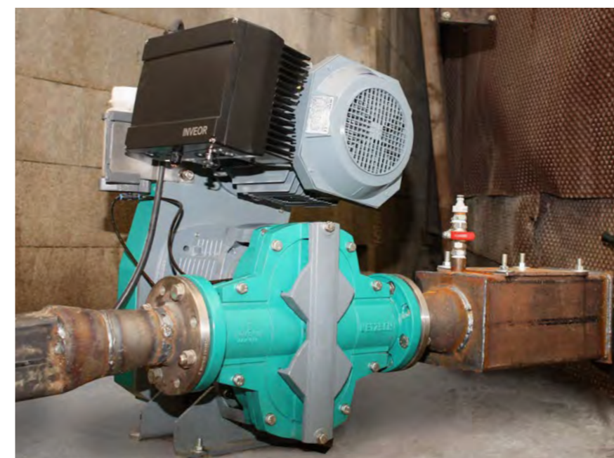
Recirculating liquid manure in a biogas plant from a fermenter to a heat exchanger at a flow rate of 20 m 3 /h against a discharge pressure of 1,5 bar.
