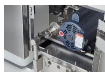
8 gpm filter pump
