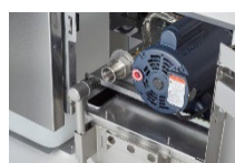
8 gpm filter pump
