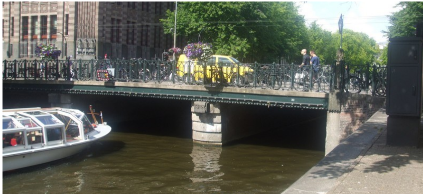
Fig. 2: One of the evaluated old bridges in Amsterdam, the Isa van Eeghenbrug
