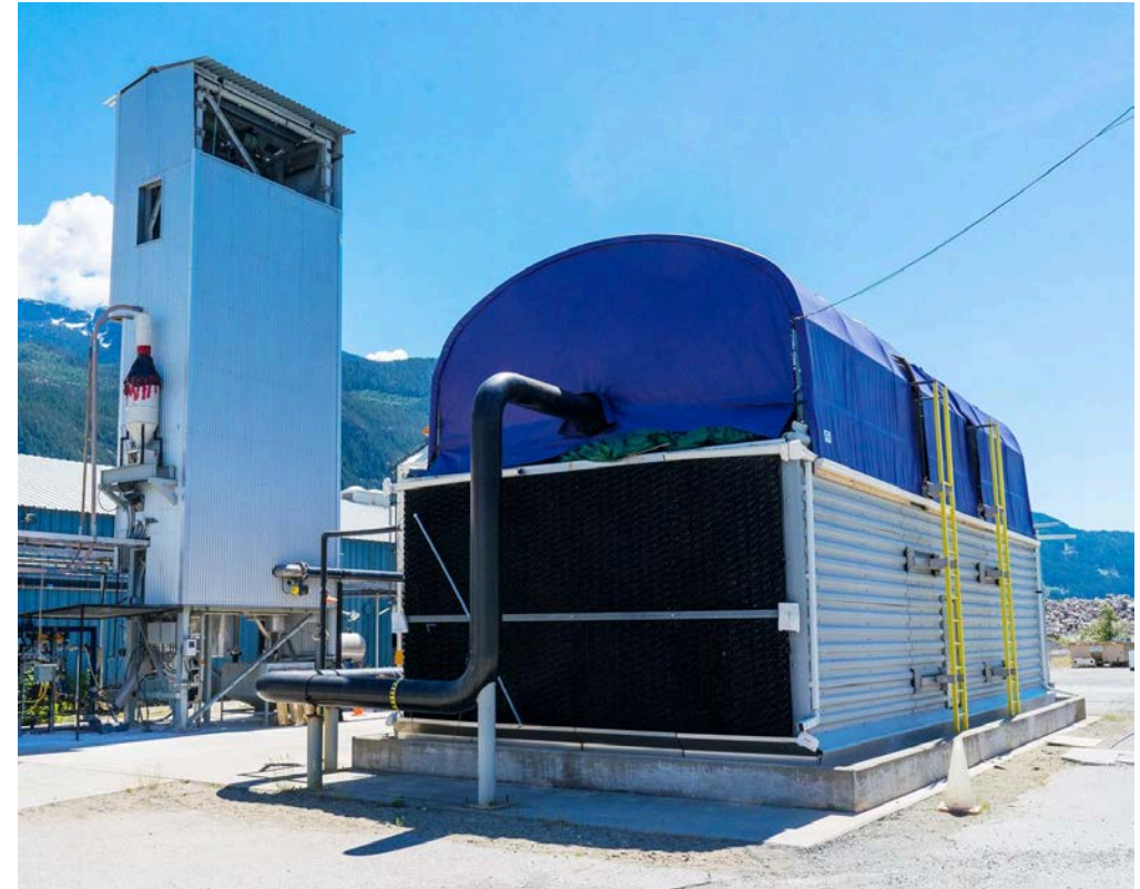
Carbon Engineering facility in British Columbia captures 1 ton/day
