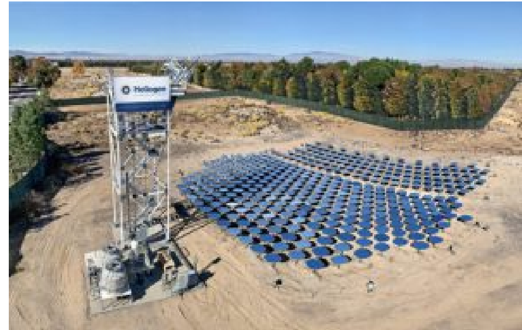
Heliogen Mirror Array in Lancaster
