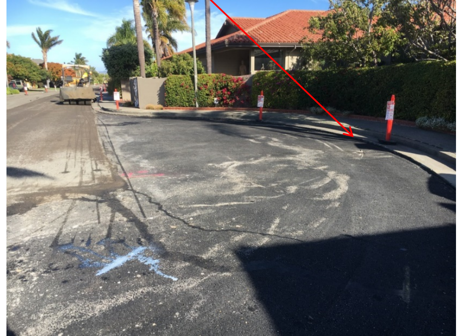
CIR Ties into new paved exterior of the cul de sac And directly to the lip of gutter.
