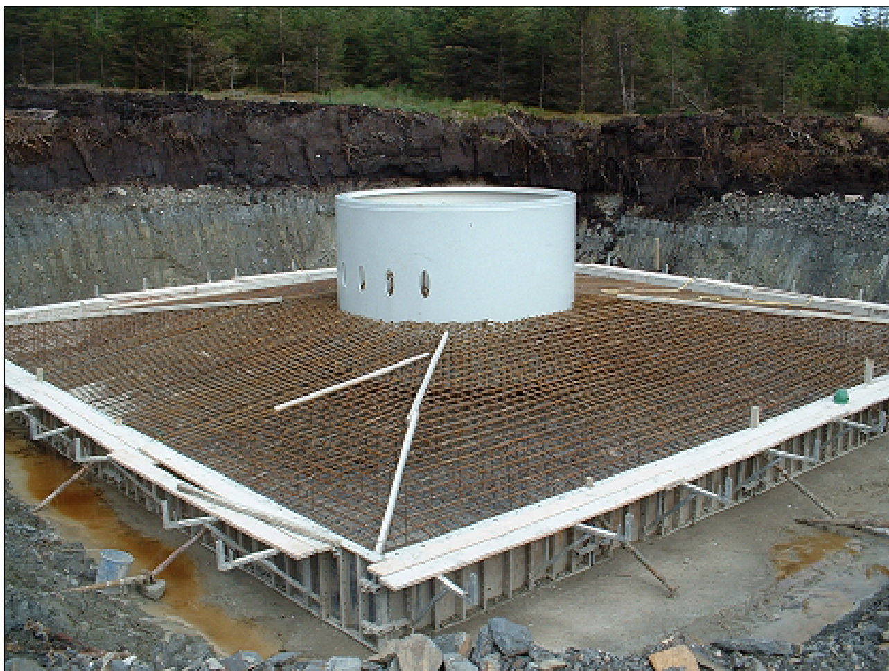
A wind turbine base at Cefn Croes, Wales, showing steel reinforcing bars and collar in place prior to pouring concrete. Note the two-metre deep peat cut through at the rear.
