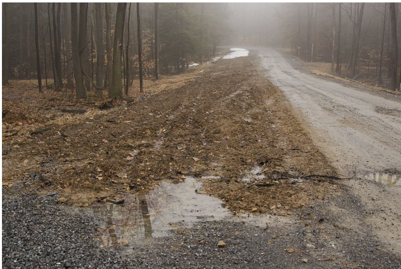
Soil that was spread on top of the gravel along this section of the road is eroding away.
