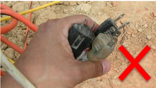
Never use extension cords that have broken or missing ground pins!
