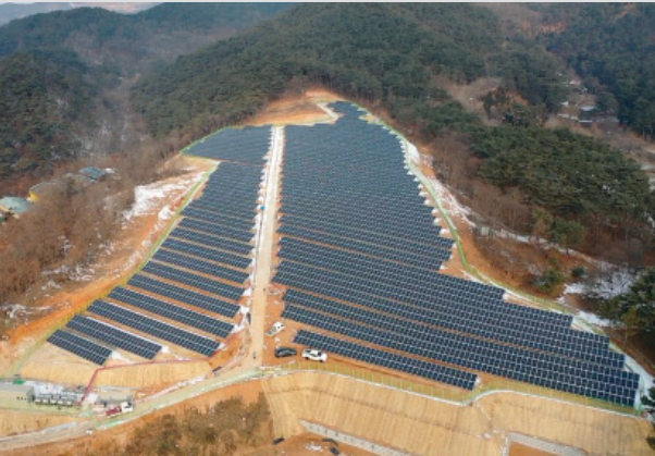
Solar Mounting Structure (Ground-Mounted Type)
