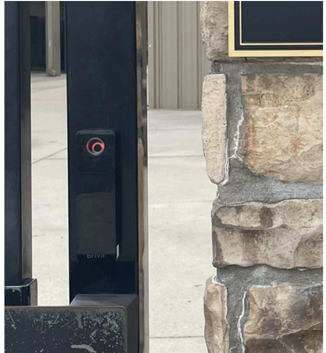
Gate Access Reader
