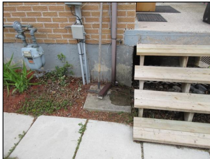
3. Discharge too close to building
