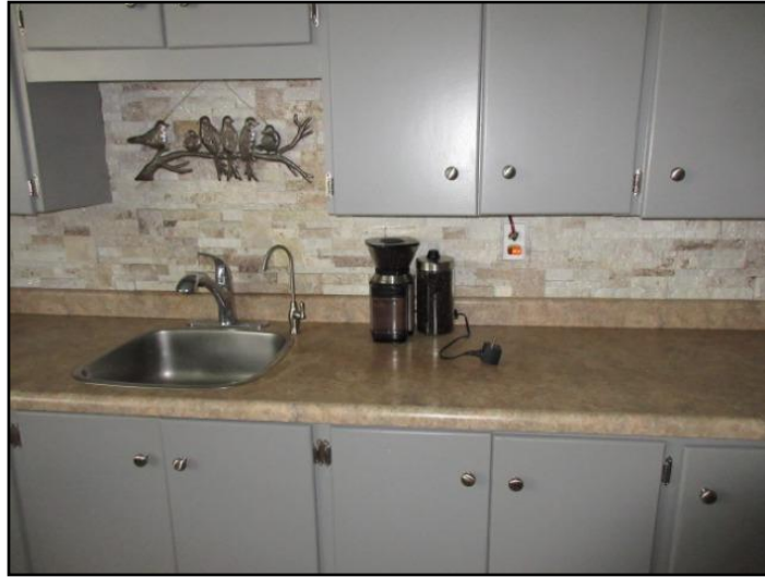
10. No GFCI/GFI (Ground Fault Circuit...
