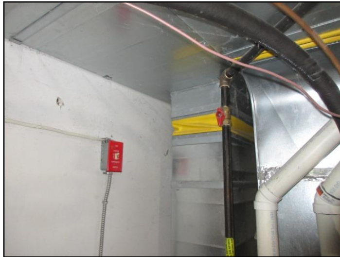
12. Main fuel shut off & electrical disconnect
