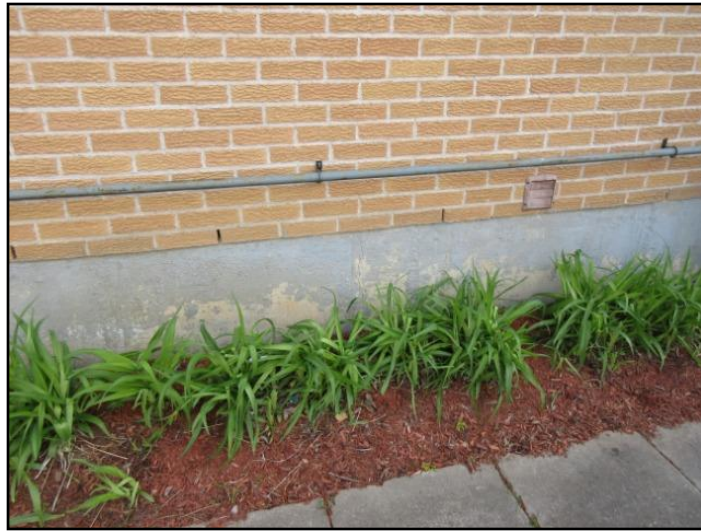
6. Typical minor cracks
