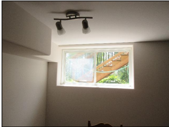
28. Lost seal on double glazing
