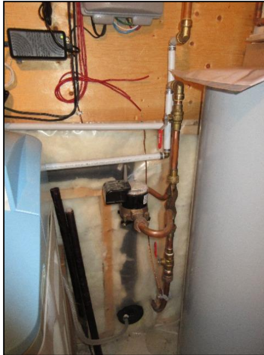
24. Main water shut off
