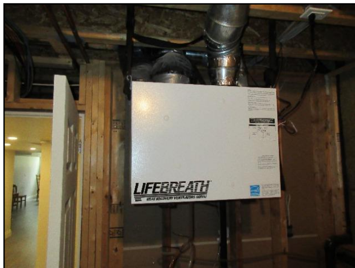
14. Heat recovery ventilator (HRV)
