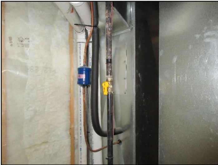
9. Main fuel shut off
