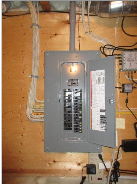
5. Main electrical disconnect
