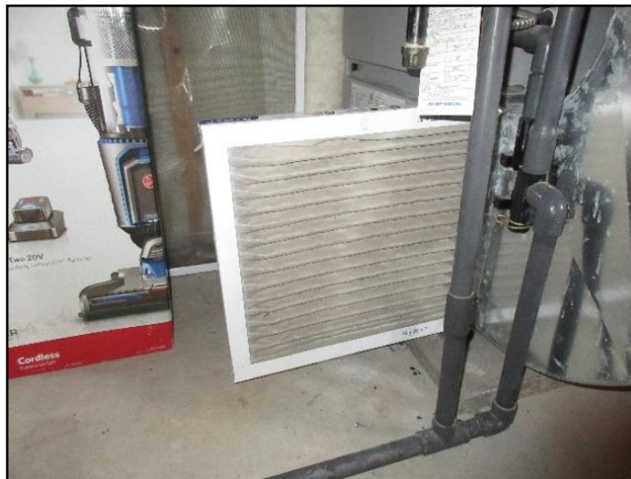
15. Replace - regular maintenance
