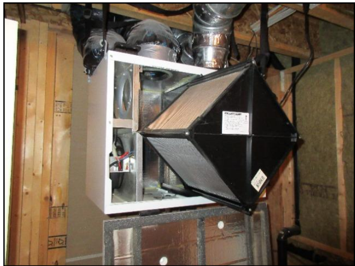
16. Clean core - regular maintenance
