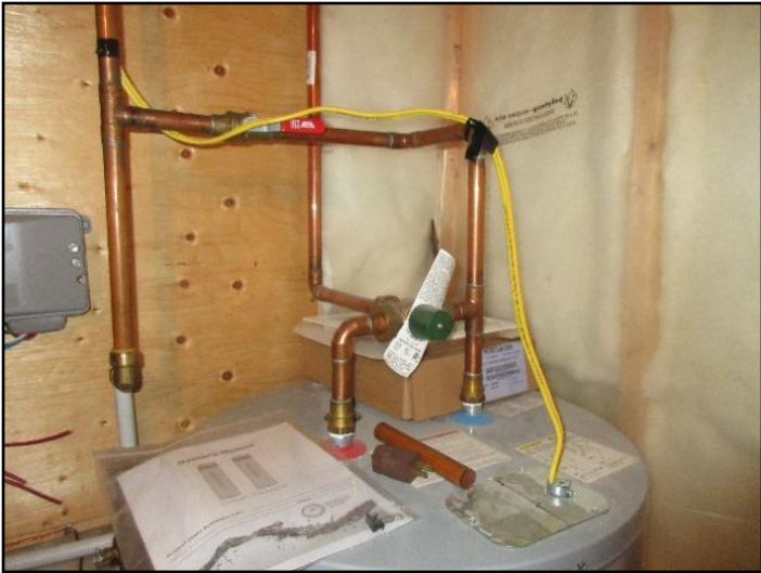
23. Tempering/mixing valve installed
