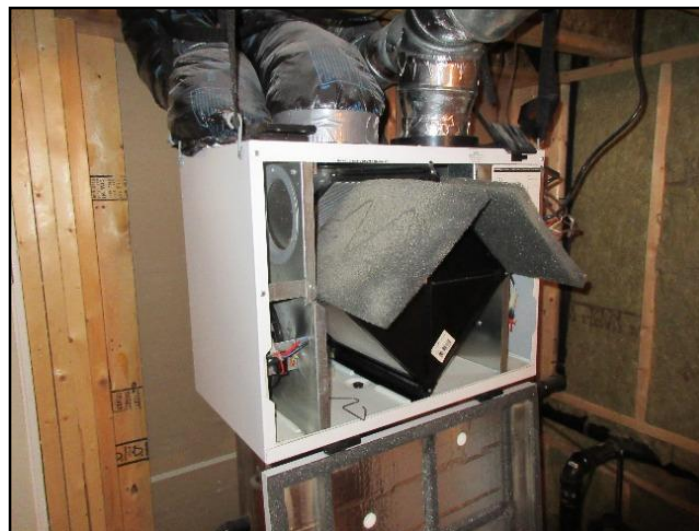
17. Clean filters - regular maintenance
