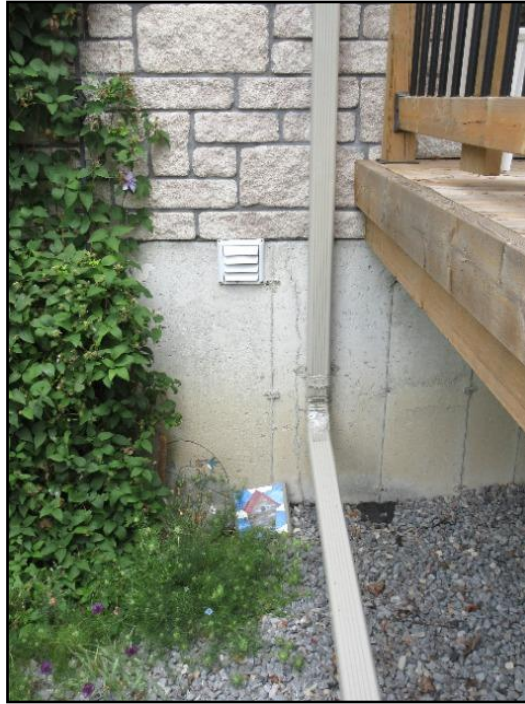
4. Typical minor cracks
