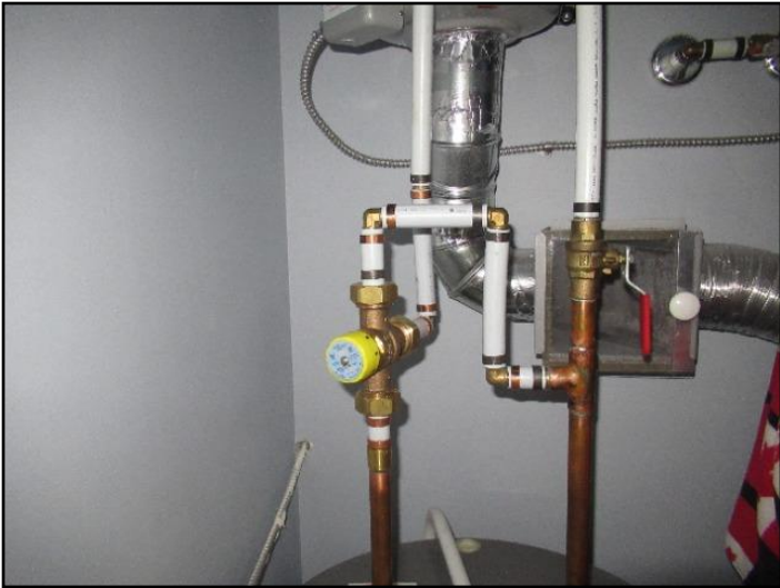
7. Tempering/mixing valve installed
