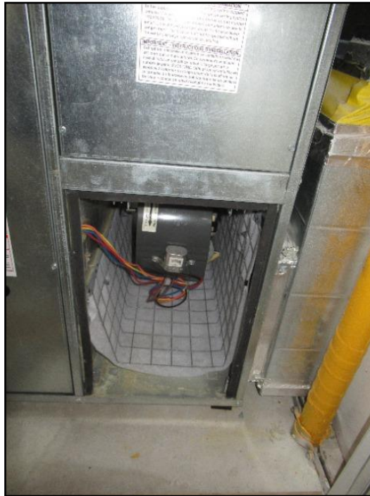
6. Replace - regular maintenance
