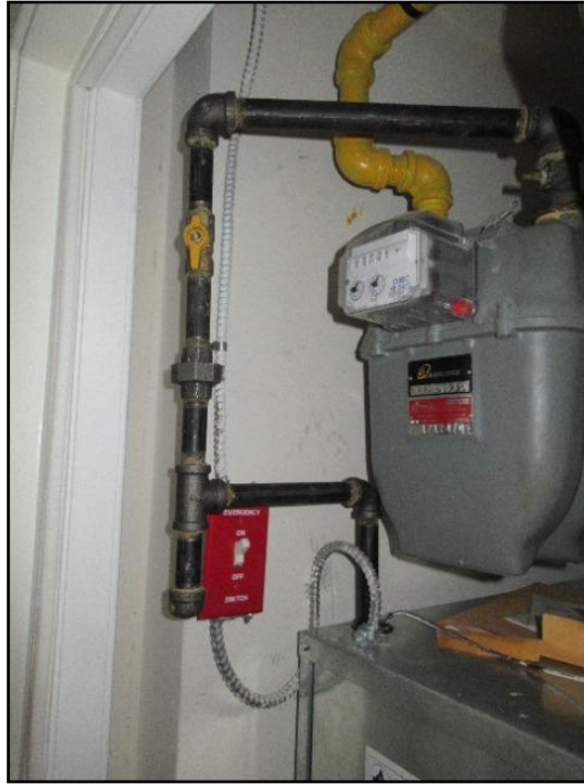
4. Main fuel shut off & electrical disconnect
