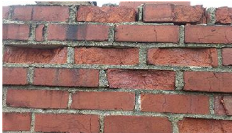
Figure 2.3 - Failing Chimney Cap
