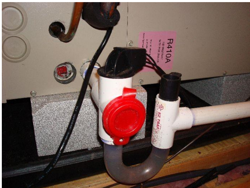
Figure 3.14 - Manufactured Trap with Safety Float Switch
