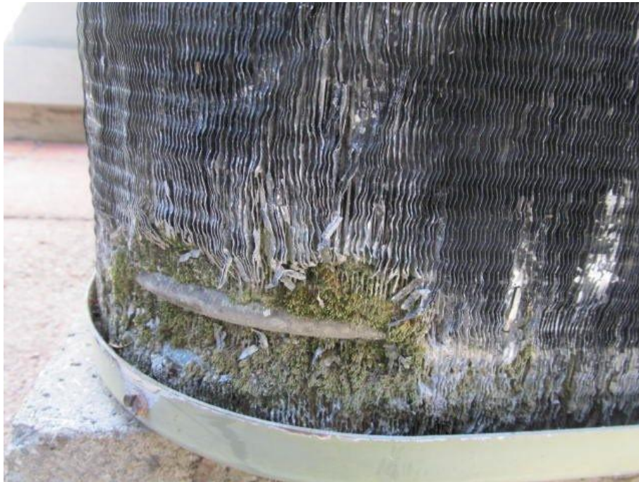
Figure 4.3 - Common Damage Found on Compressors
