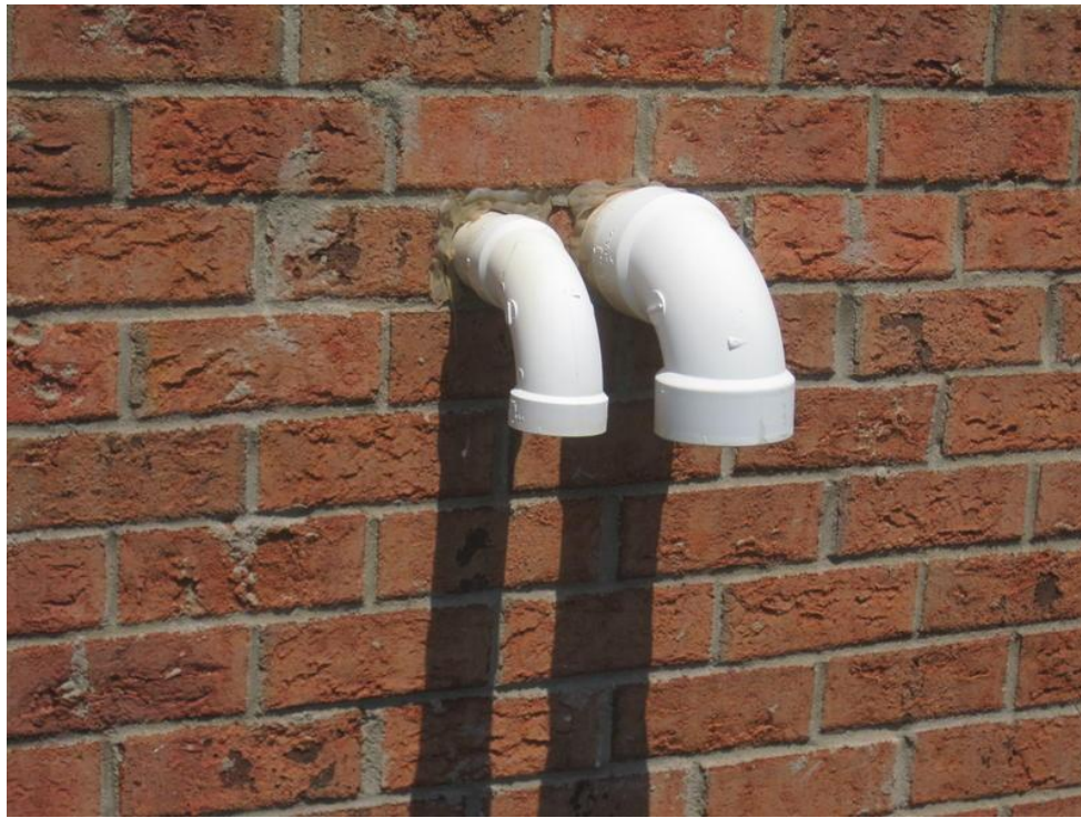
Figure 2.10 - Suspect High Efficiency System Intake / Exhaust
