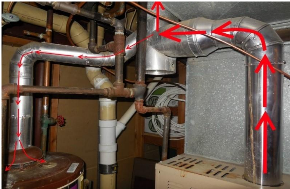
Figure 2.12 - Improper Exhaust Pairing and Exhaust Slope
