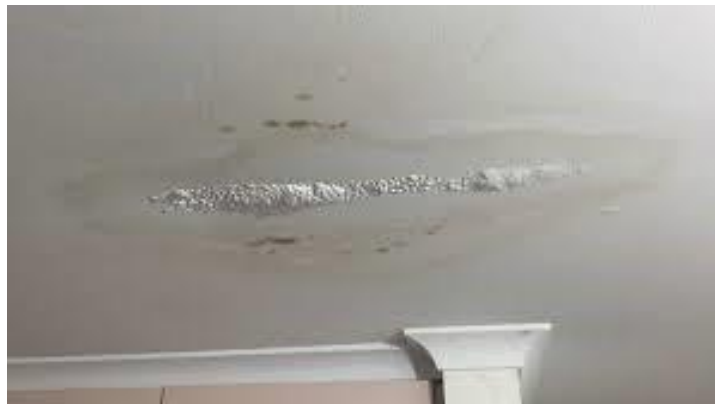
Figure 4.6 - Extensive Ceiling Damage from Failure to Install Secondary Drain Line
