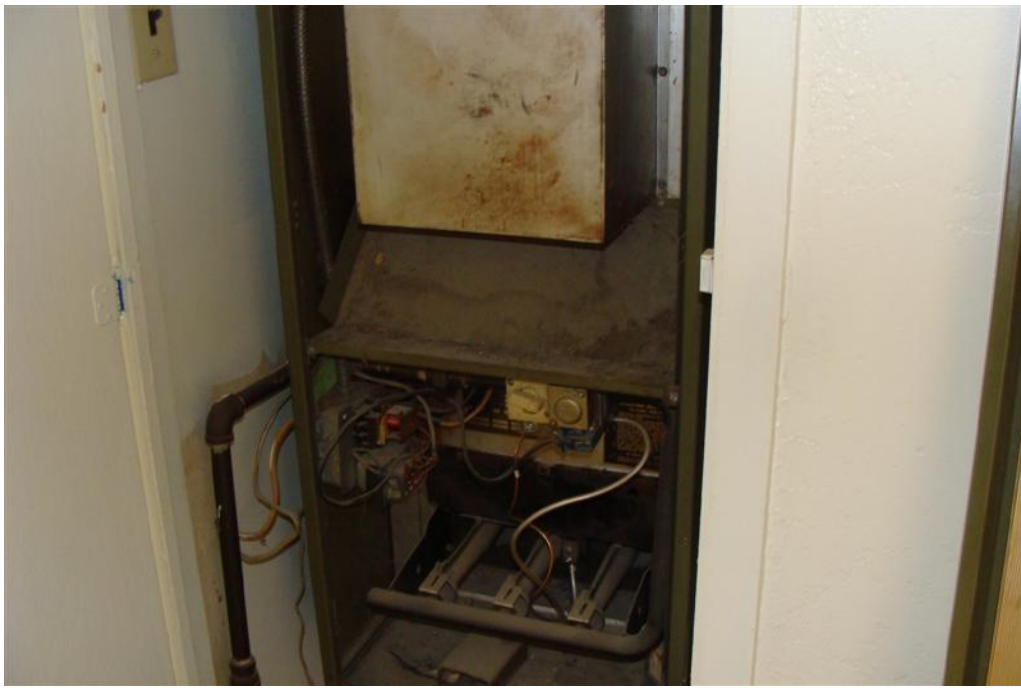
Figure 2.6 - A Seriously Scorched System Interior
