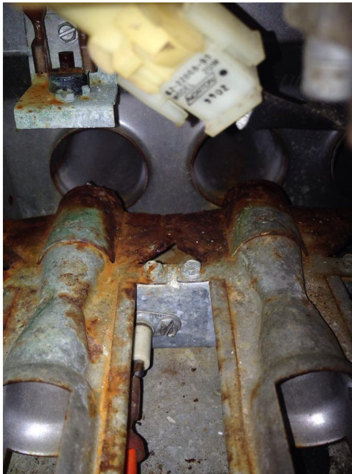
Figure 3.12 - Rust and Corrosion Damage from Clogged Condensate Drain
