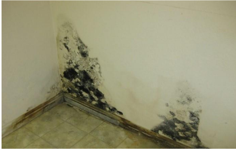
Figure 4.7 - Structural Damage from Failure to Monitor Proper Drainage
