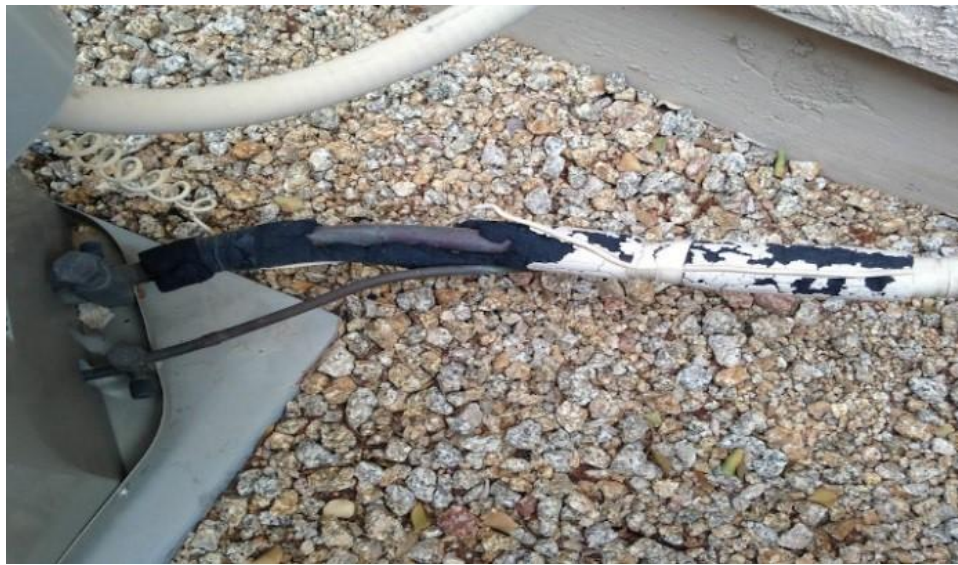
Figure 4.4 - Refrigerant Line Insulation Decay
