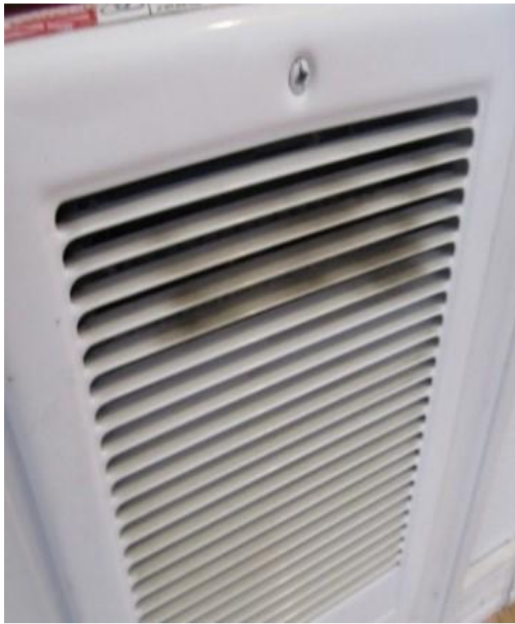
Figure 2.4 - Scorched Register Observed in Room
