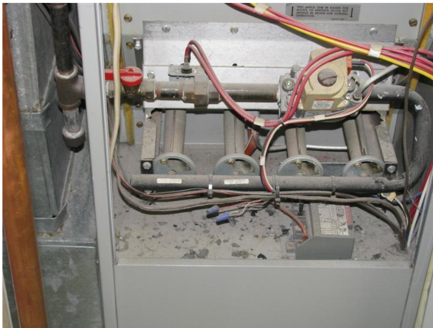
Figure 3.10 - Improper Fuel Supply Manual Shut-Off
