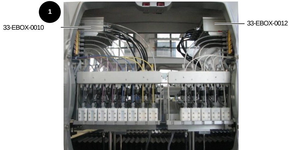
Top Right teh – Internal View
