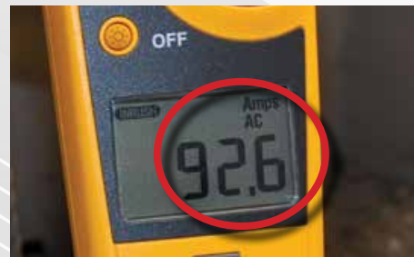
Amp measurement without 5-2-1 ® Compressor Saver ®
