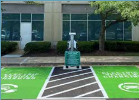
Electric Vehicle Charging Stations
