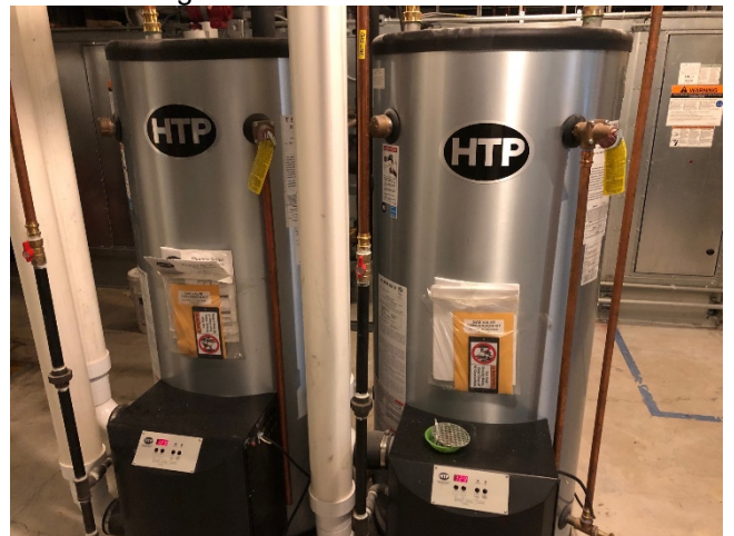
Hot Water Heaters
