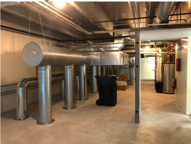
Mezzanine Level Mechanical Room
