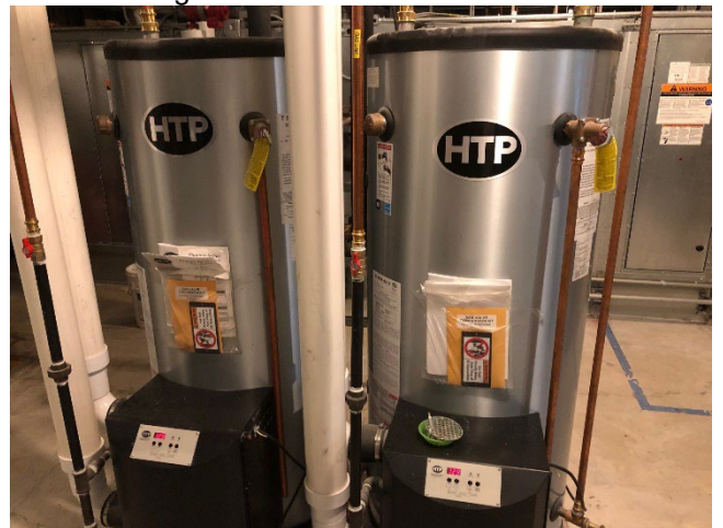
Hot Water Heaters
