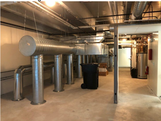
Mezzanine Level Mechanical Room
