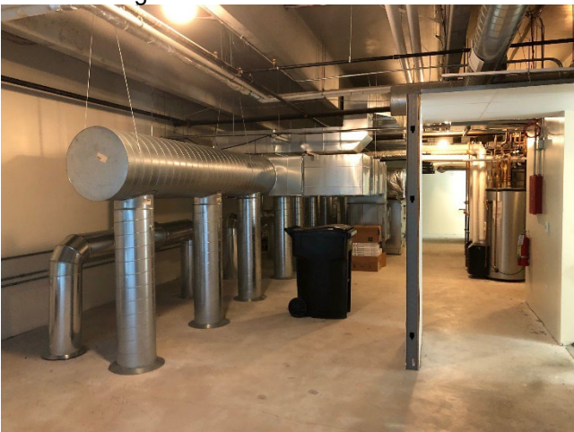
Mezzanine Level Mechanical Room
