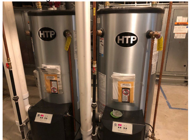
Hot Water Heaters
