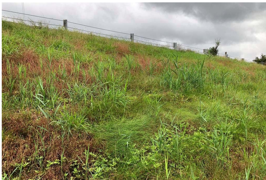
Picture 9 – Saturated area at the NE corner.
