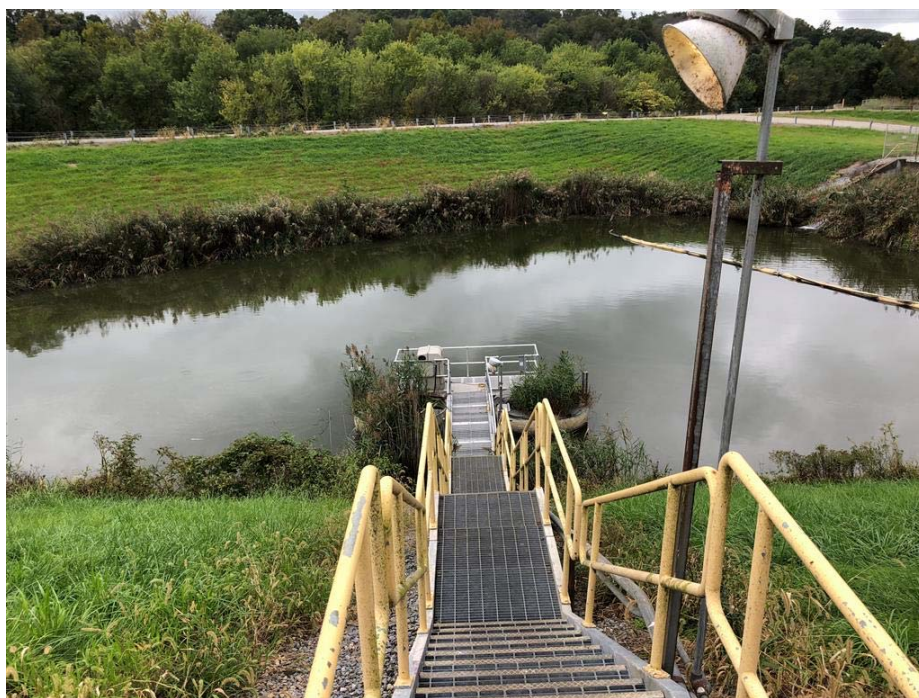
Picture 12 – Vegetation should be removed from the risers.
