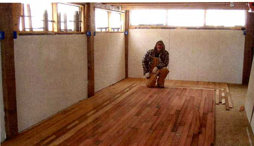
Fancy. The palace parquet won't look out of place, because the rest of the barn's flooring is fancy, too. Here, I'm installing madrone flooring with an oak surround (all salvaged stock, of course).
