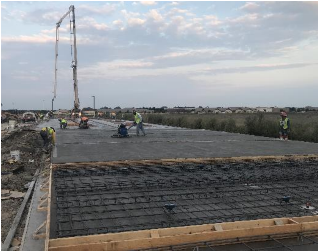
Fig. 4 (from Part 1): Panels in various stages, a) Finishing of poured panels, b) Panel ready for pour
