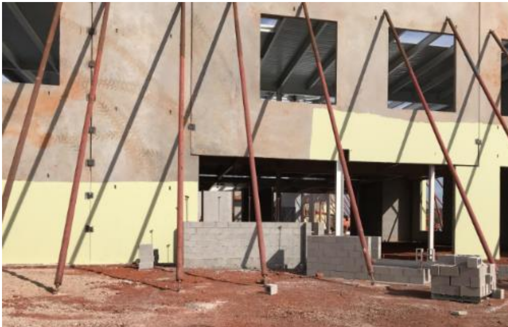
Fig. 61, Panel opening too wide below. Panel supported by adjacent panels.
