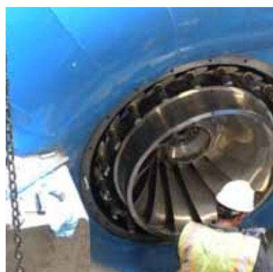
ABIQUIU HYDROPOWER PROJECT 2009-2011 Uses 50/50 public-private funding for low-flow turbine | NM
