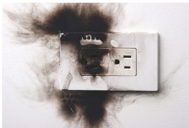
Scorch marks on cover plate
