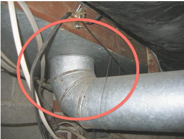
Loose connection; recommend sealing.
