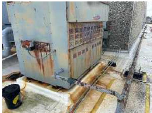
Gas piping to rooftop boiler
