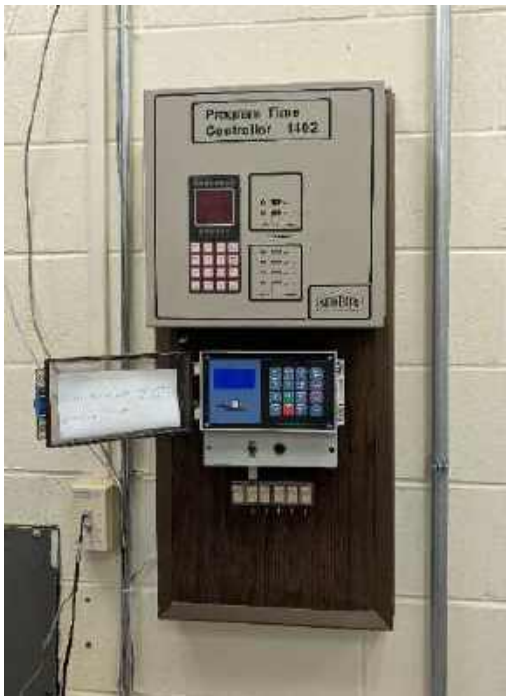
BAS Controller in Main Office
