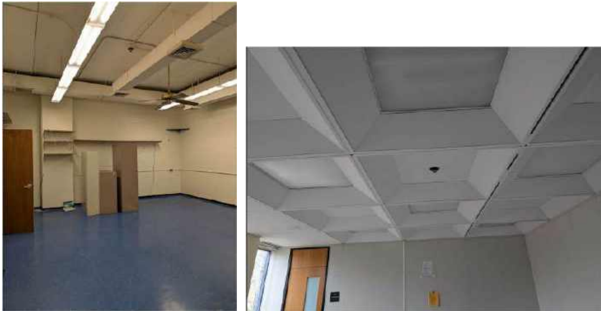
Typical Pendant and Troffer Fluorescent Fixtures with No Sensors Visible
