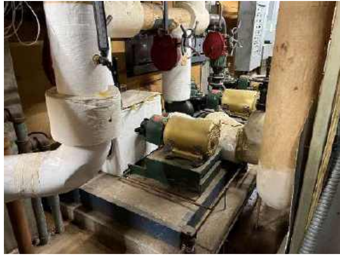
Condenser Water Pumps
