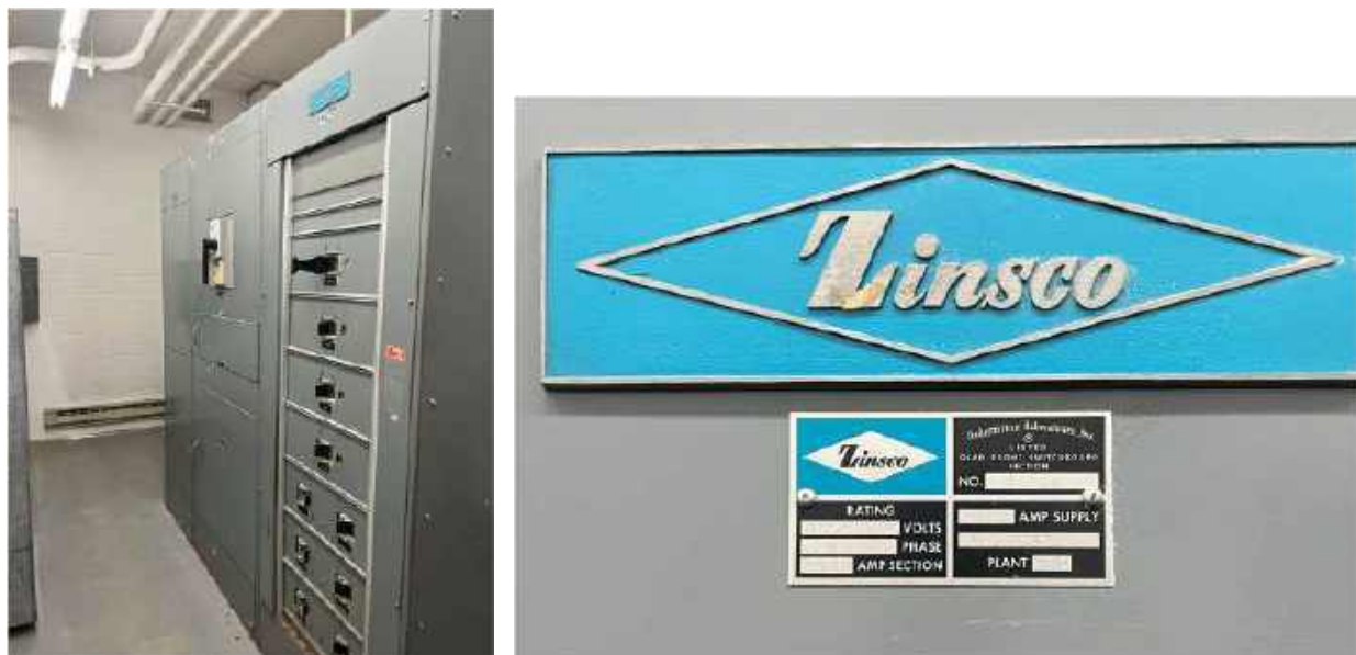
Existing 2500A 480Y/277V Zinsco Switchboard and Nameplate
