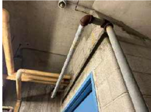
Galvanized Steel Vent Piping
