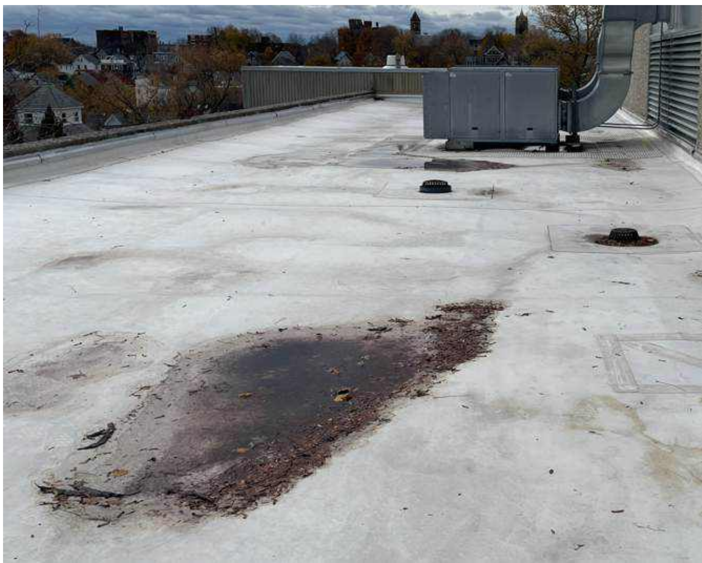
Ponding and soft roof from possible moisture below membrane
