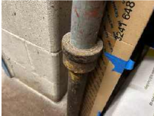
Cast Iron Sanitary Drain Piping
