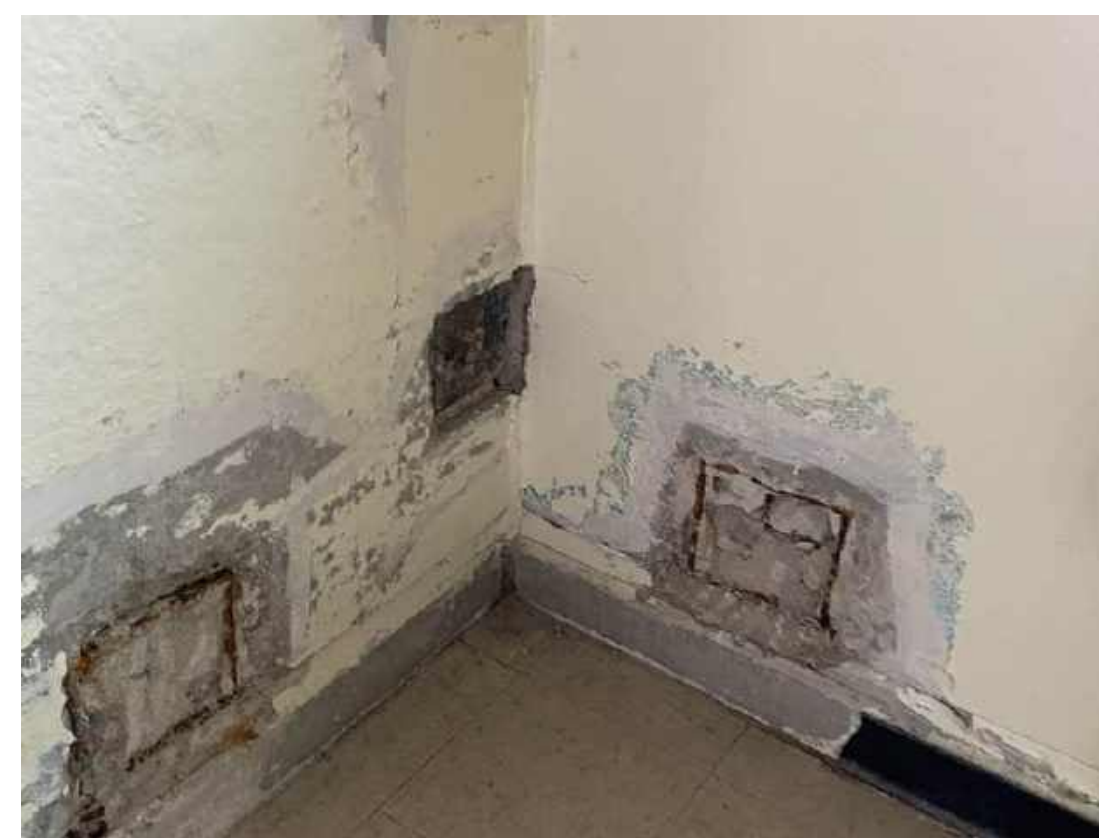
Stairwell Walls Spalling Concrete/Exposed Reinforcing
