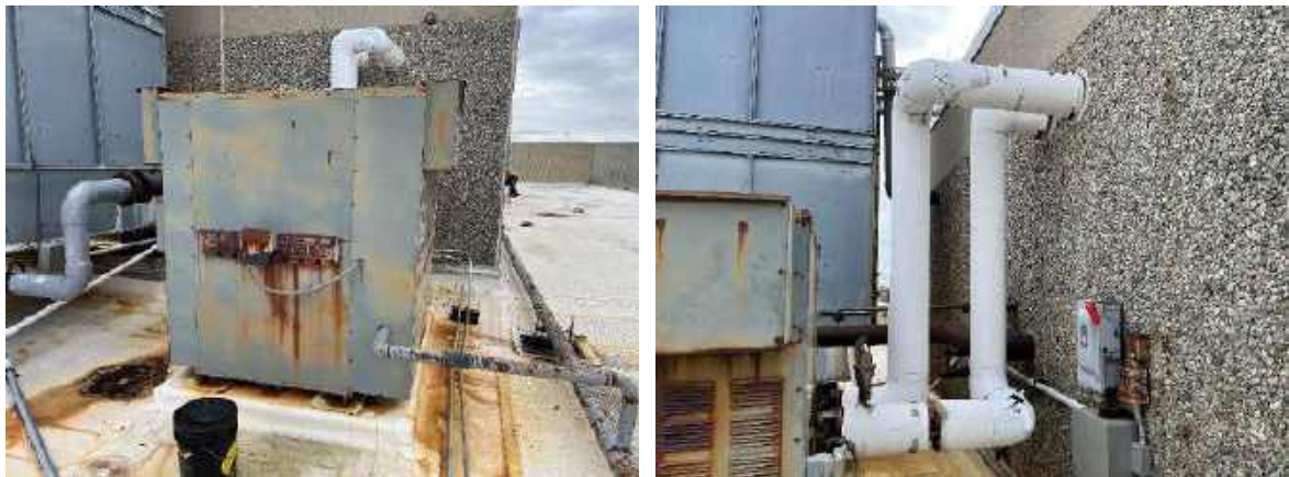
Natural Gas Boiler and Hot Water Piping into Mechanical Penthouse
