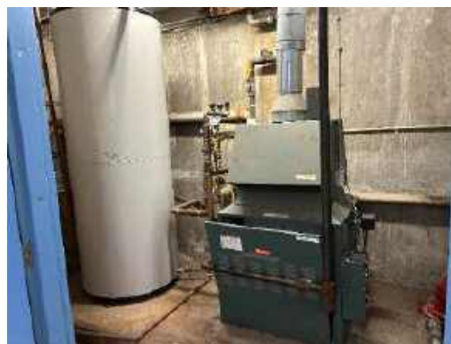
Water Heater & Storage Tank
