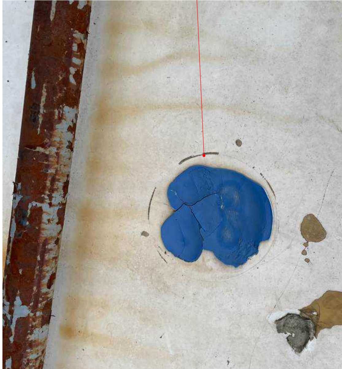
Patch in Roof leaks
