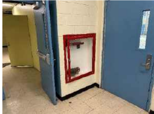
Photo 2- Standpipe Valve Cabinet
