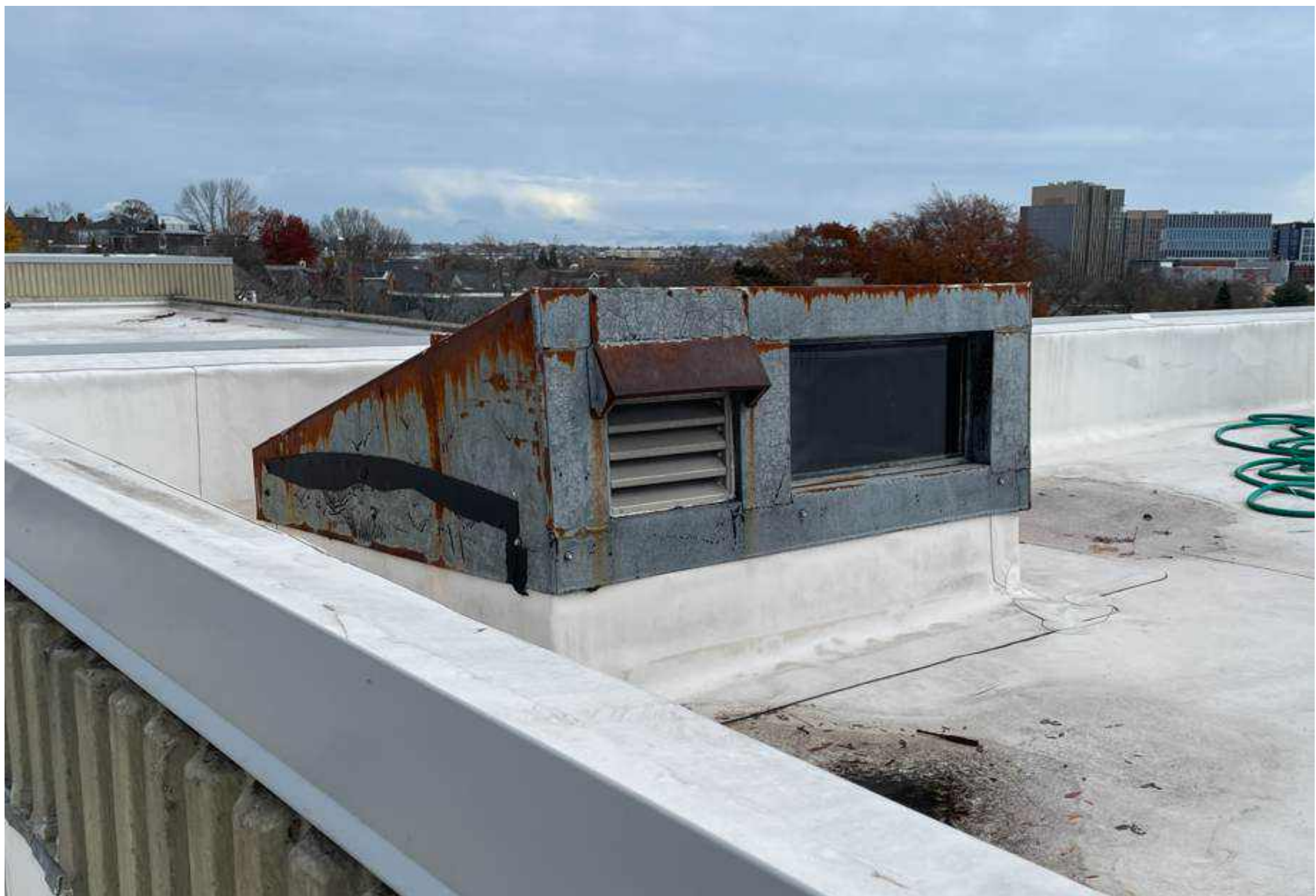
Outdated and rusty mechanical intake
