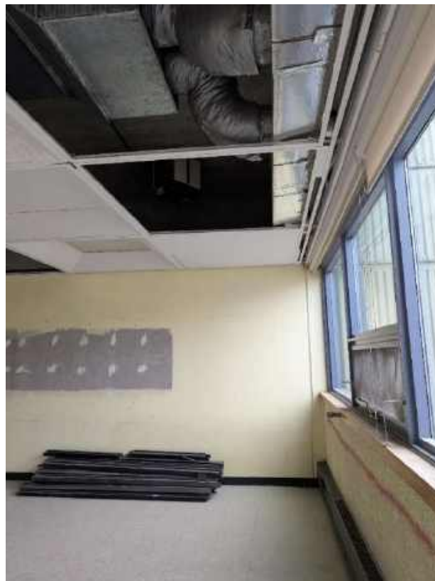
Classroom with Perimeter Electric Baseboard Heating, Linear Diffusers for Ventilation, and Return Plenum with electric heater
