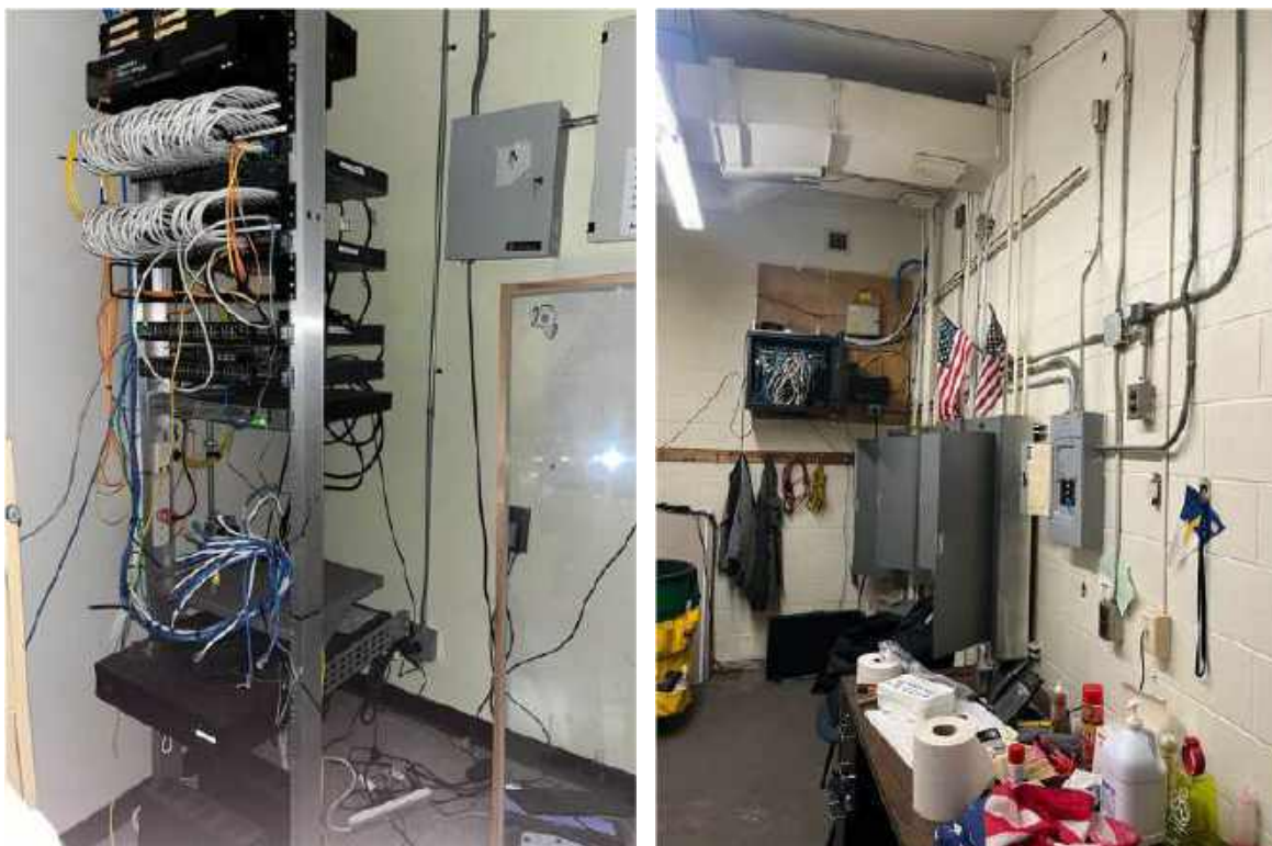
MDF within admin storage (left) and Trapeze Rack in Custodial Room (right)
