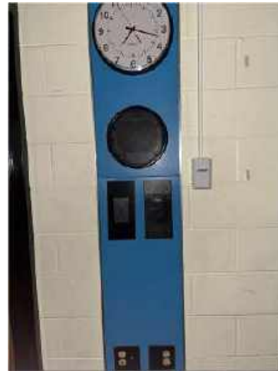
Typical Electrical Media Panel
