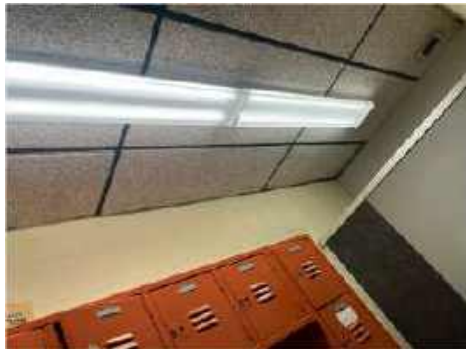
Locker Room Fixtures
