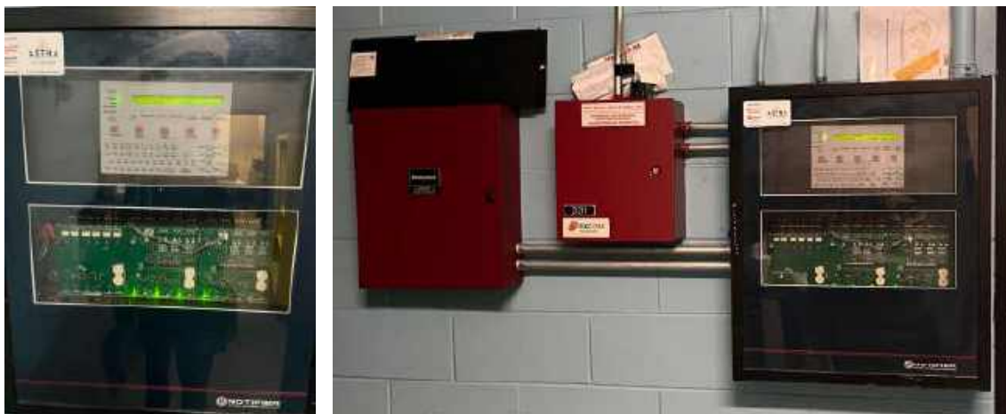
Honeywell – Notifier Fire Alarm Control Panel, Power Supply, and FD Comms Device
