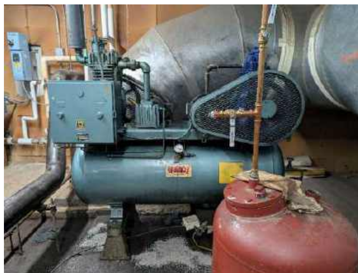
Air Compressor serving Pneumatic Controls
