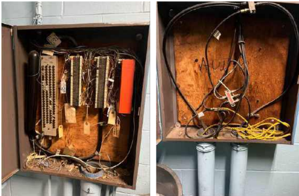
Verizon Phone Main Cabinet (Left) and Audio Visual Main Cabinet (Right)
