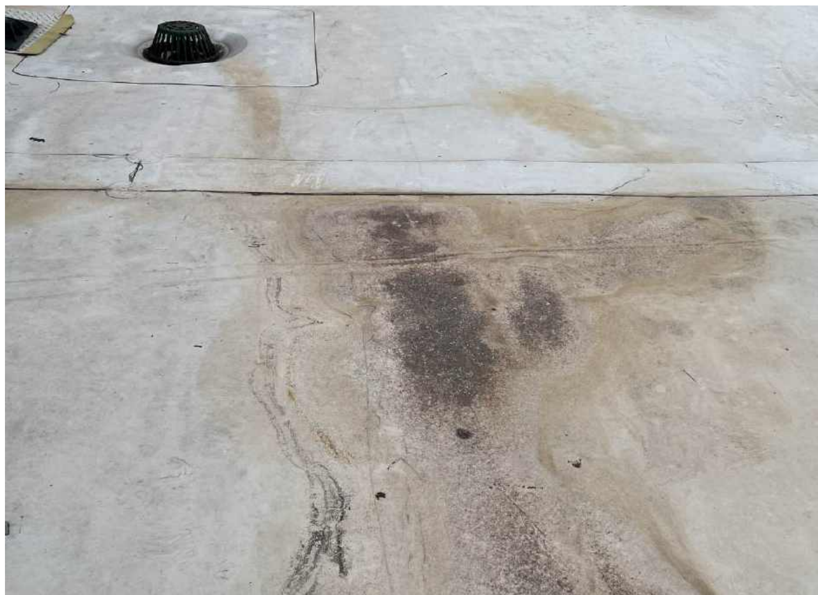
Ponding and soft roof from possible moisture below membrane
