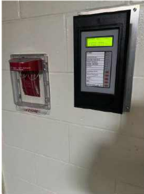
Annunciator and Covered Fire Alarm Pull Station
