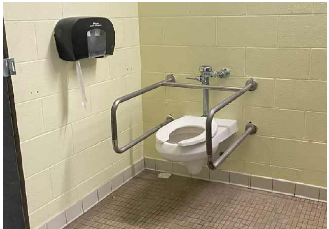
Non-Compliant grab bars and toilet accessories
