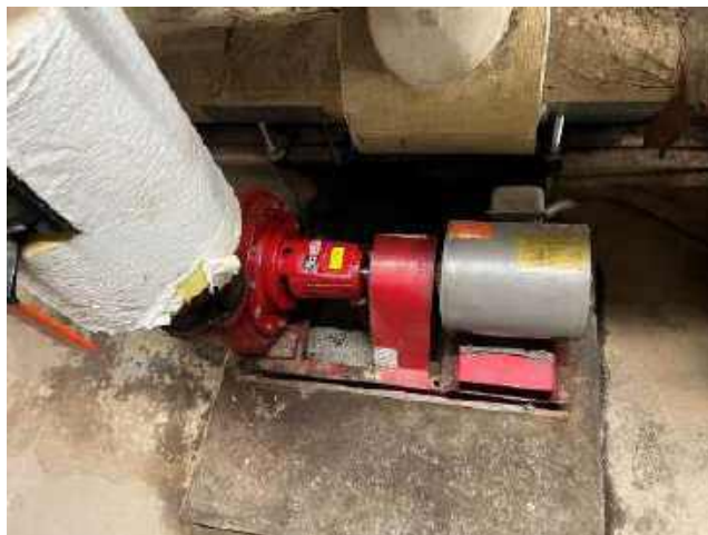
Hot Water Pump
