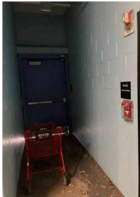
Pull Station Greater than 5 ft within Exit Door, Not Code Compliant
