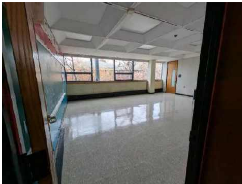
Typical Classroom with Perimeter Electric Baseboard Heating, Ventilation via Linear Diffusers along Modular Tiles
