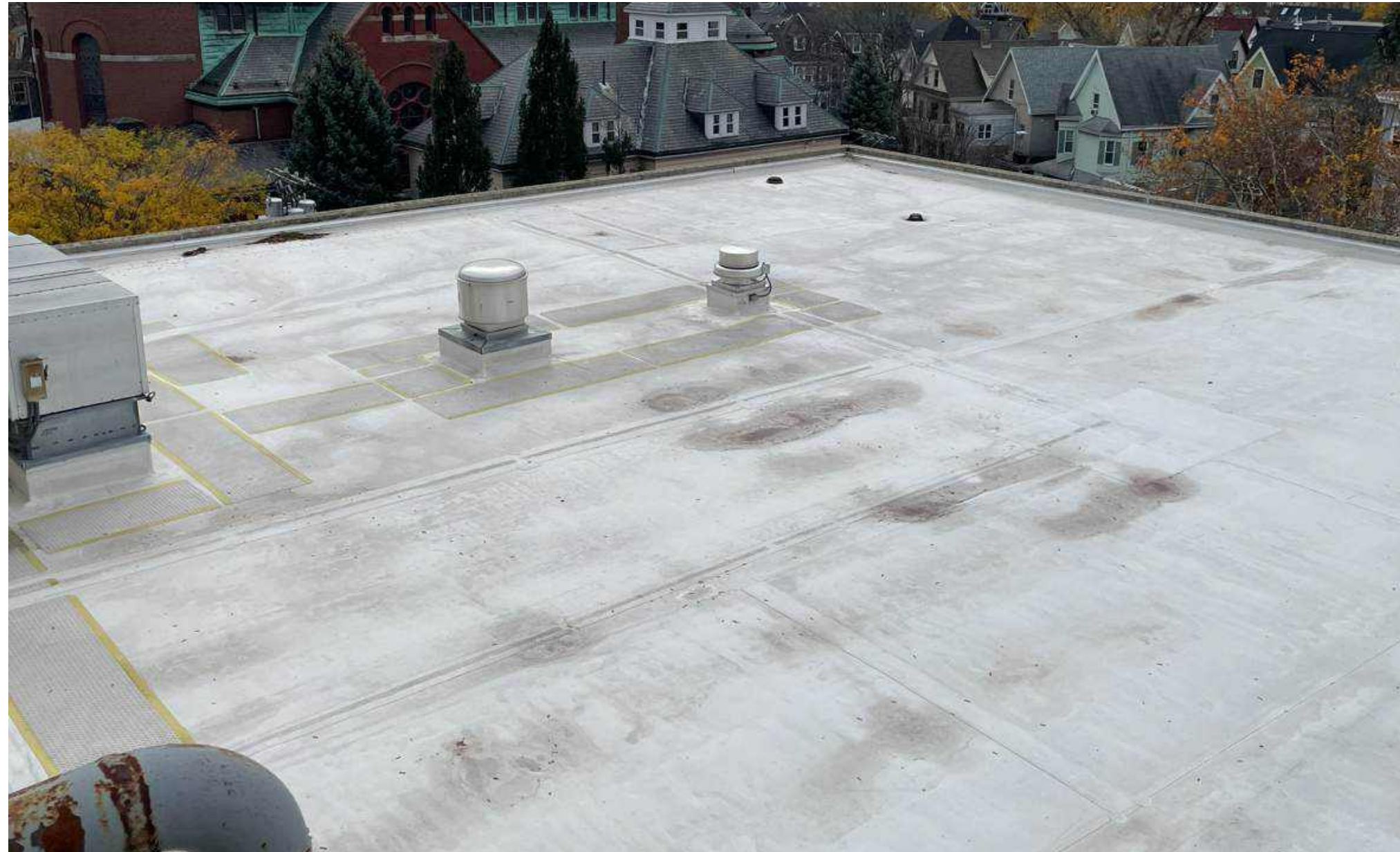
Gymnasium Roof Lacks Roof Drains
