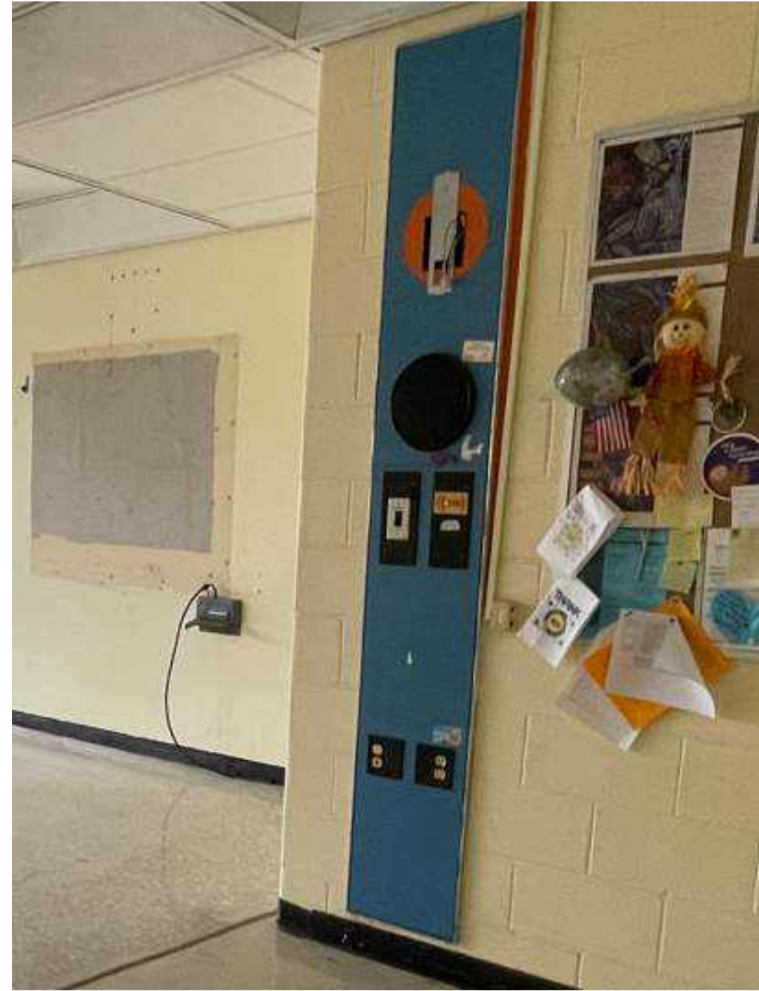
Classroom Control Panel
