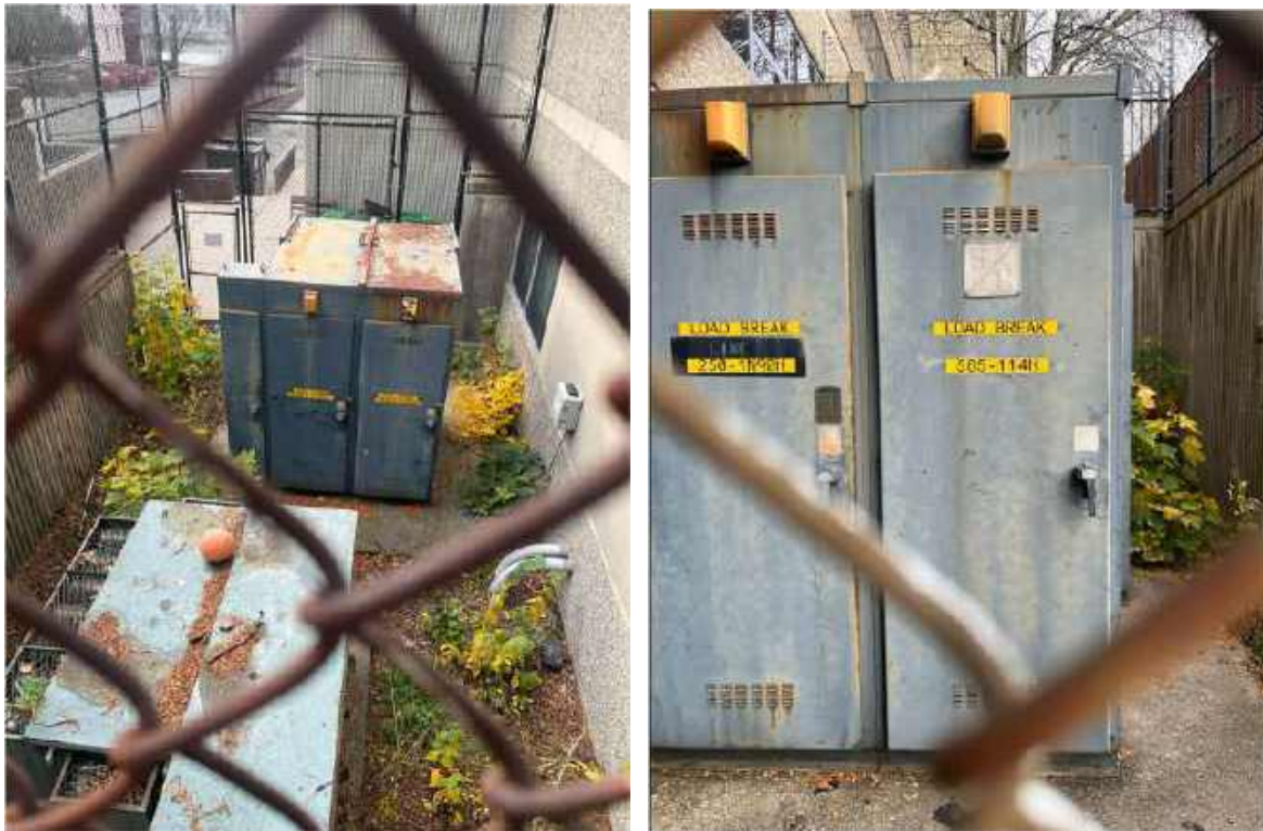
The 13.8kV Utility Load Breaker and Primary Utility Transformer Enclosure
