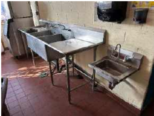
Prep and Handwash Sinks
