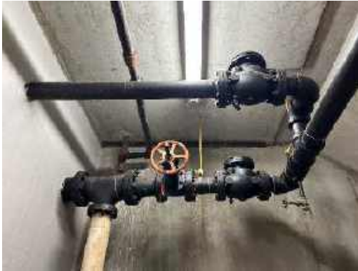
Photo 1- Incoming Fire Service & FDC
