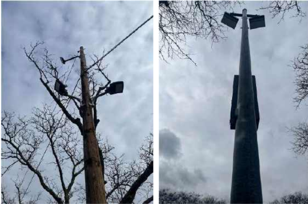
Exterior site lighting poles
