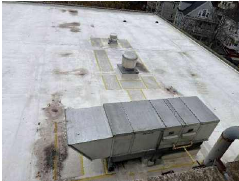
Gas-Fired Heating Only RTU and Exhaust Fans on Lower Gym Roof
