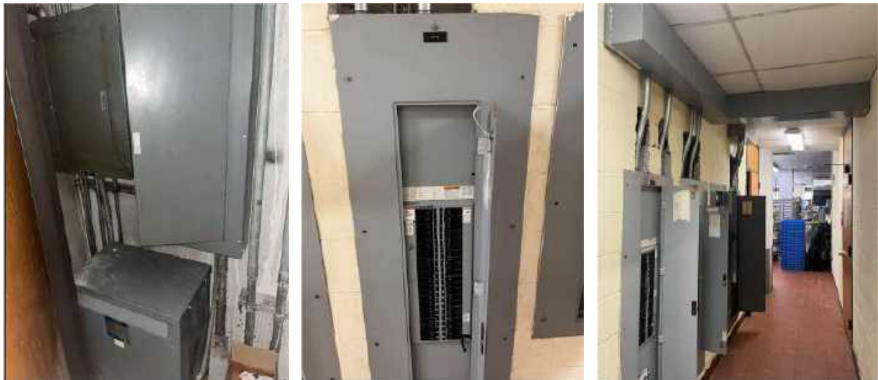
Examples Of Typical Riser Closet Panelboards and Kitchen Panels
