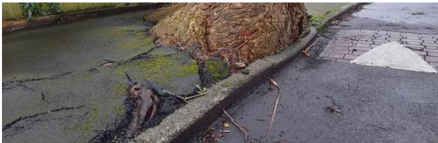
Figure 5. Insufficient subsurface growing space exposes roots. Photo Credit: Manx Roots Tree Management.
