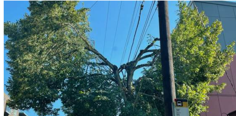
Figure 6. Utility Infrastructure conflicts with canopy. Photo Credit: West Street Blog
