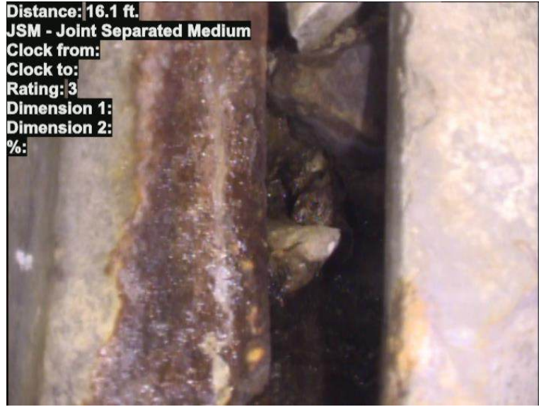
FIGURE 5: JOINT SEPARATION WITH INFILTRATION IN STORM DRAIN 7-5831 : 7-5829
