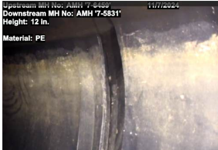
FIGURE 3: JOINT SEPARATION IN STORM DRAIN 7-6459 : 7-5831
