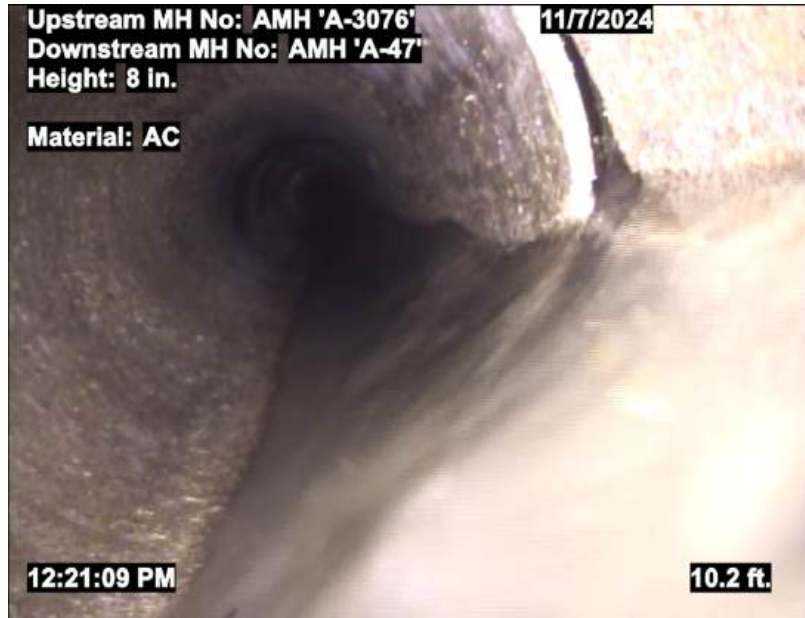
FIGURE 1: JOINT OFFSET IN SANITARY SEWER MAIN A-3076 : A-47
