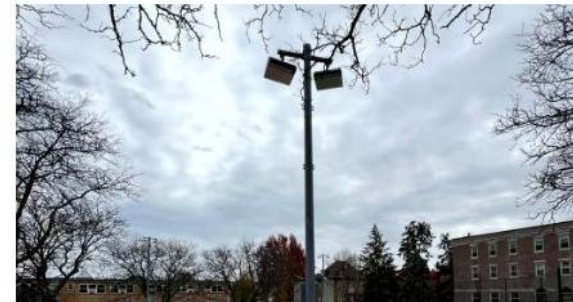
FIELD LIGHT Quantity: 4 Condition: Fair
