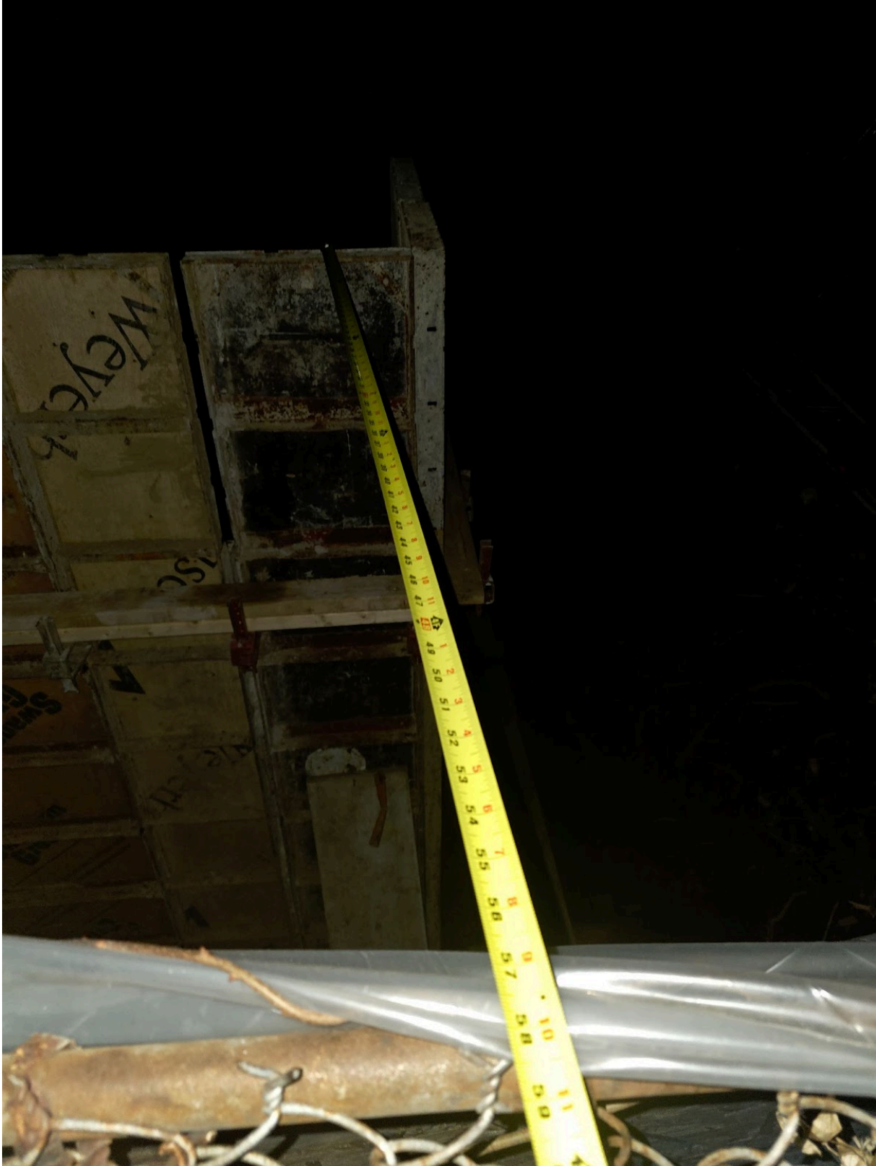
Measurement from the edge of the forms to the fence shows 58 inches.
