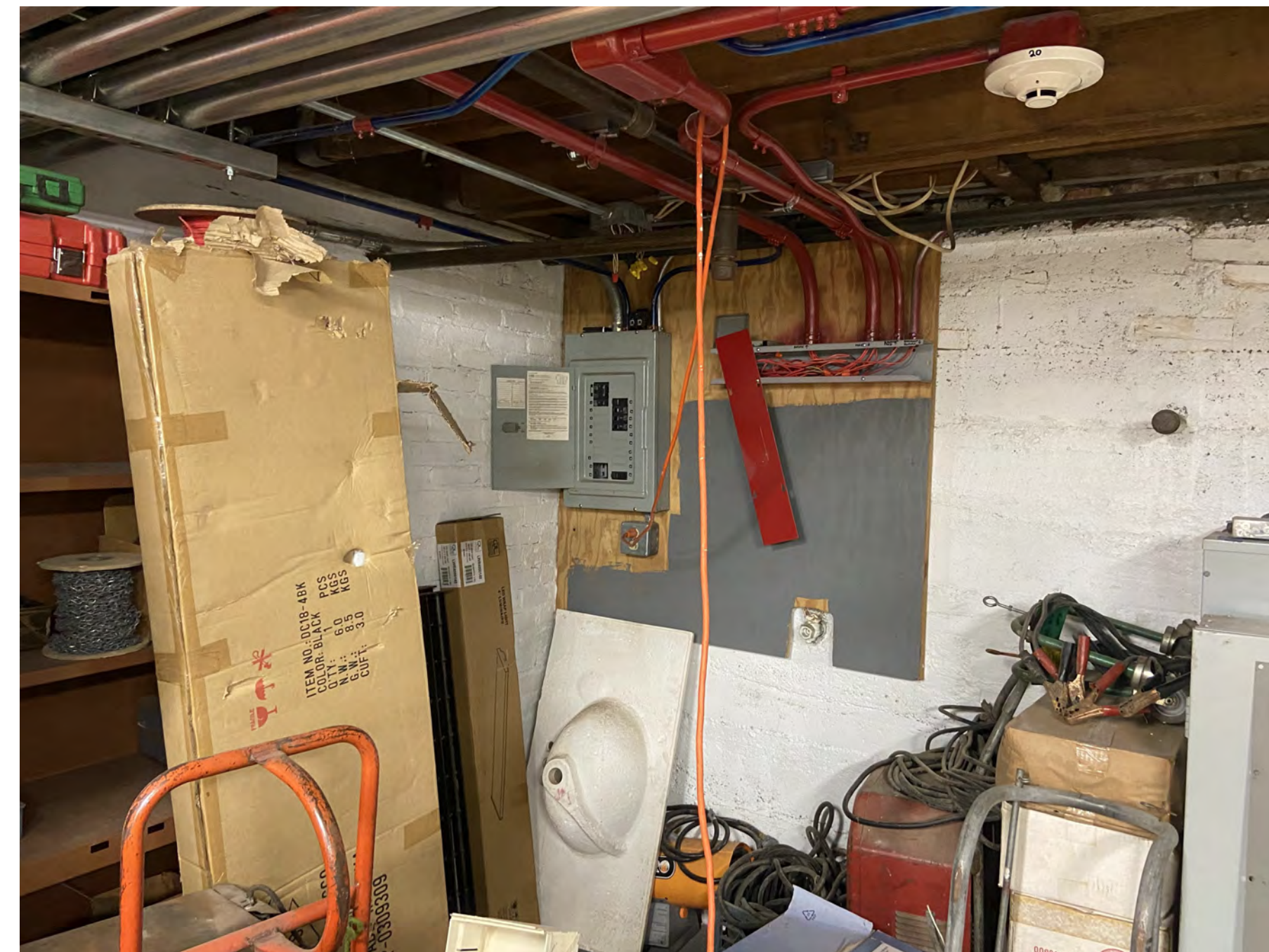
ENLARGED PHOTO SHOWING ELECTRIC PANEL, FIRE ALARM BUS / CONDUIT AND ELECTRICAL DISTRIBUTION THAT WOULD NEED TO BE RELOCATED AS PART OF FULL COMPLIANCE PLAN
