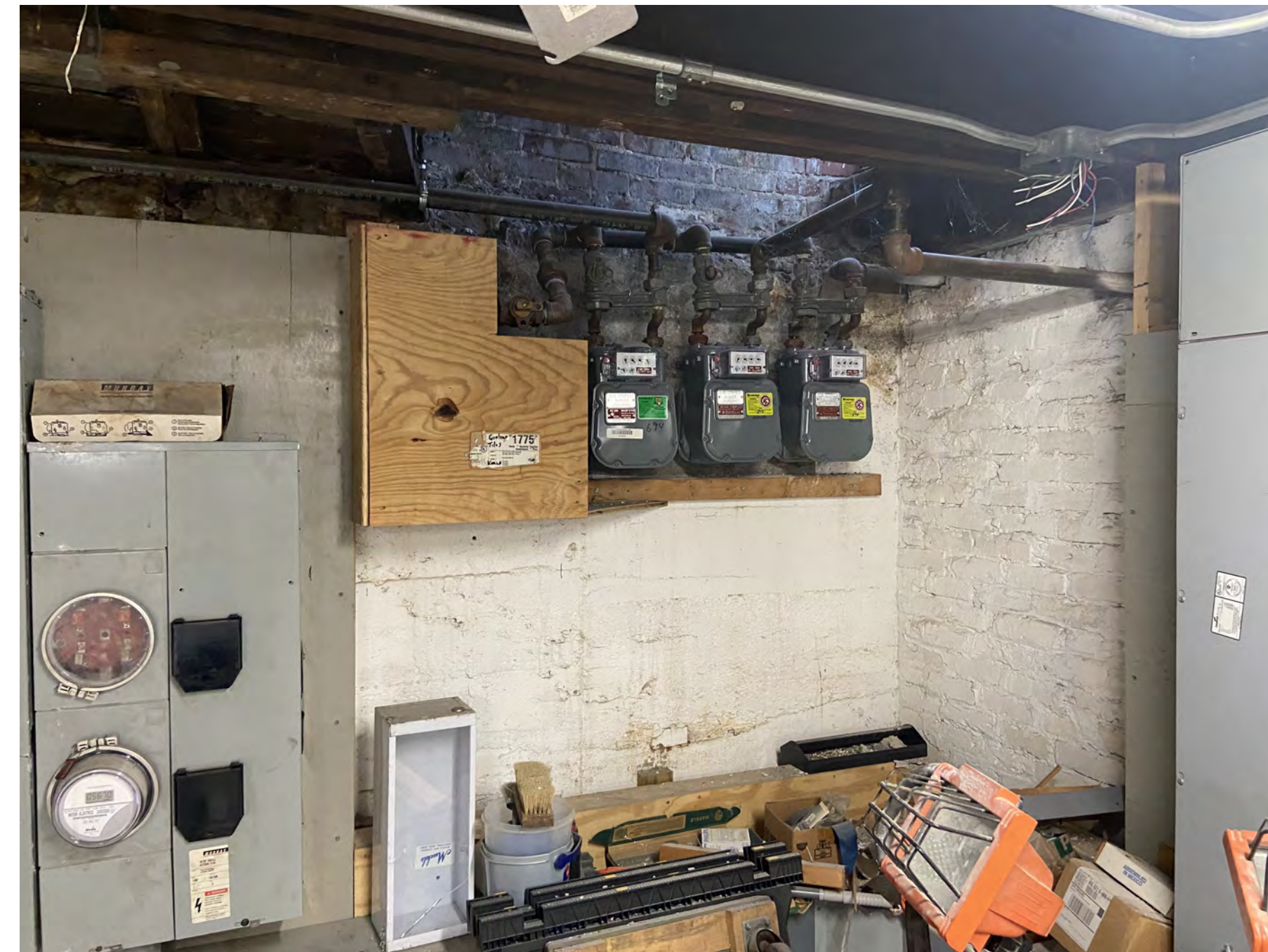
ENLARGED PHOTO SHOWING THE METERS, MAINS, AND UTILITY CONNECTIONS TO THE STREET THAT WOULD NEED TO BE RELOCATED AS PART OF FULL COMPLIANCE PLAN
