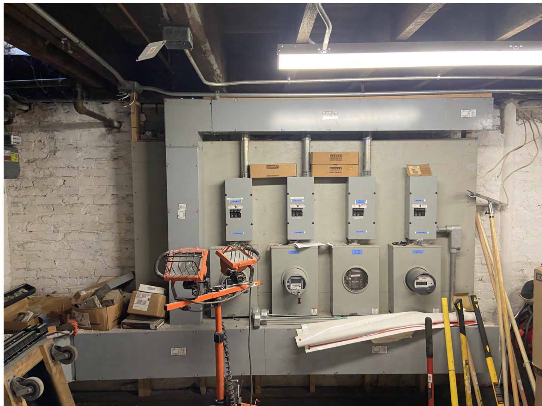
ENLARGED PHOTO SHOWING THE METERS AND ELECTRICAL BUS THAT WOULD NEED TO BE RELOCATED AS PART OF FULL COMPLIANCE PLAN
