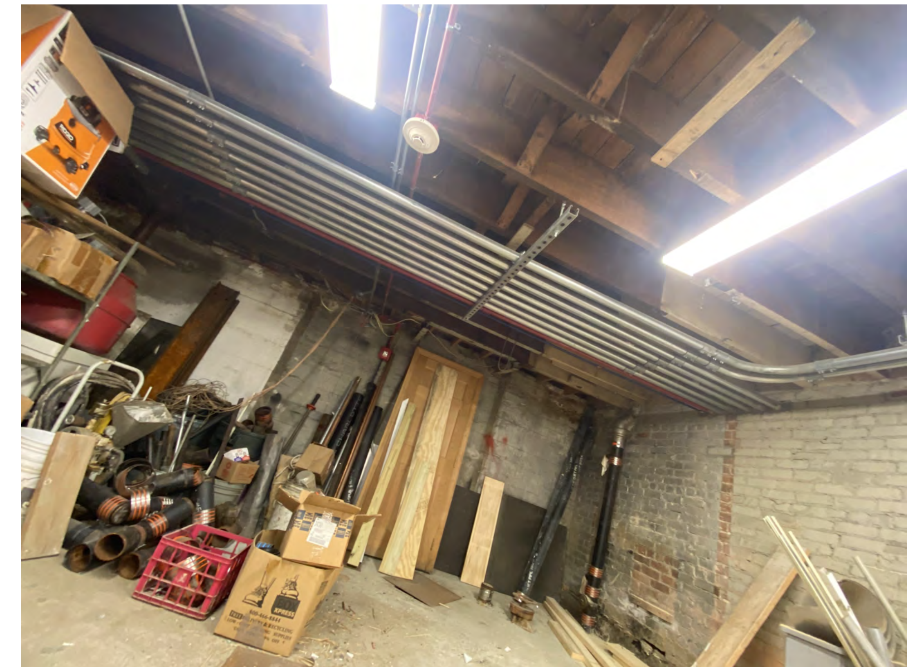
ENLARGED PHOTO SHOWING FIRE ALARM CONDUIT AND ELECTRICAL DISTRIBUTION THAT WOULD NEED TO BE RELOCATED TO LOWER THE FLOOR FRAMING AS PART OF FULL COMPLIANCE PLAN
