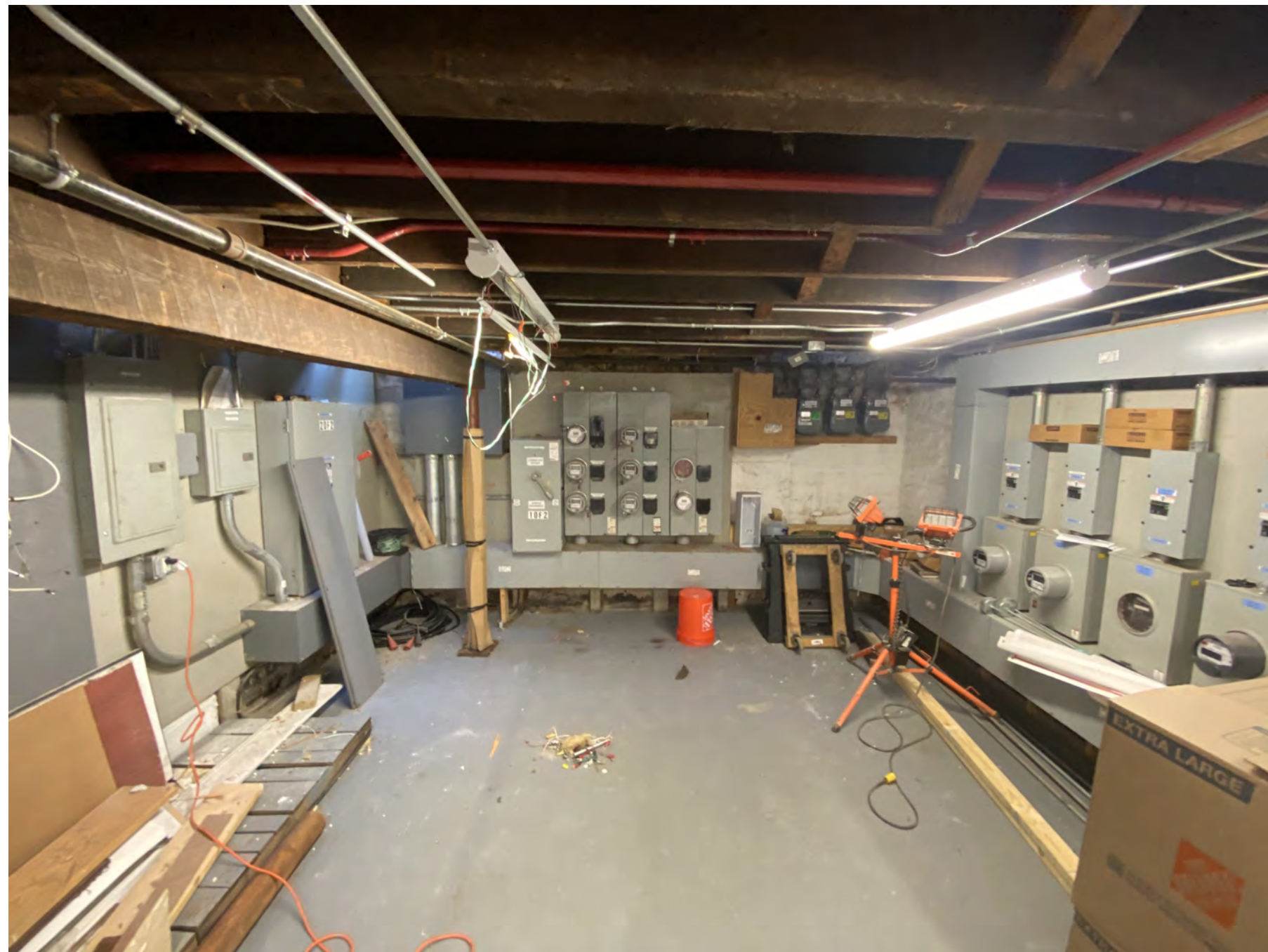
PARTIAL VIEW OF BASEMENT SHOWING EQUIPMENT THAT WOULD NEED TO BE RELOCATED AS PART OF FULL COMPLIANCE PLAN
