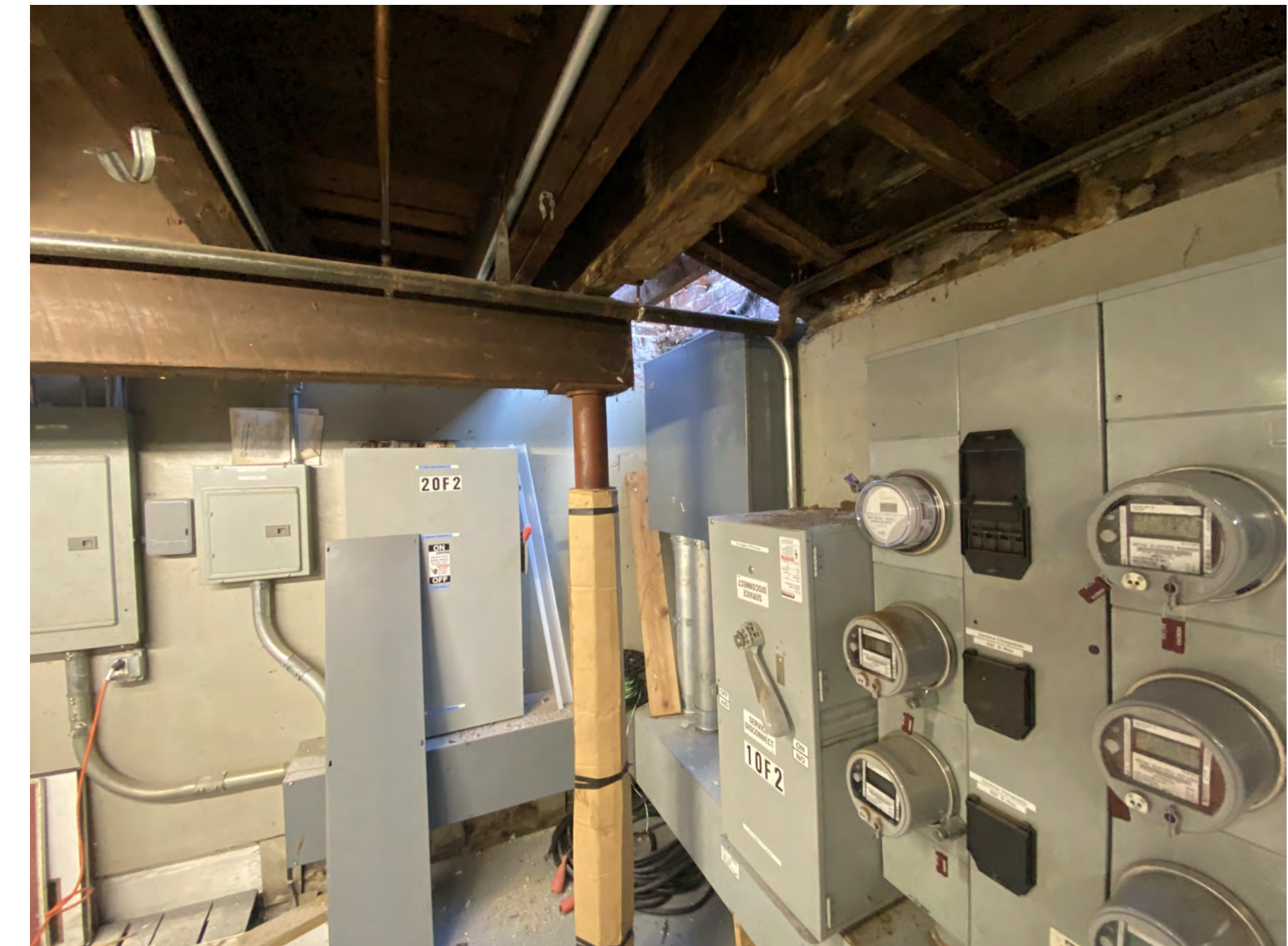
ENLARGED PHOTO SHOWING THE METERS, MAINS, AND UTILITY CONNECTIONS TO THE STREET THAT WOULD NEED TO BE RELOCATED AS PART OF FULL COMPLIANCE PLAN. ADDITIONALLY, A NEW FOOTING WOULD NEED TO BE POURED, THE STRUCTURE SHORED AND SUPPORTED, THE LALLY COLUMN RELOCATED, THE FLOOR FRAMING CUT BACK AND RE-FRAMED
