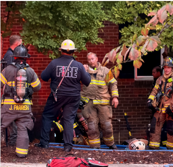
EMMA PERMAN | STAFF PHOTOGRAPHER Emergency personnel respond to a fire after an insulation caught fire as crews completed plumbing work in a crawl space Sept. 23 at E apartments. The apartments are currently vacant as they undergo a remodel.
