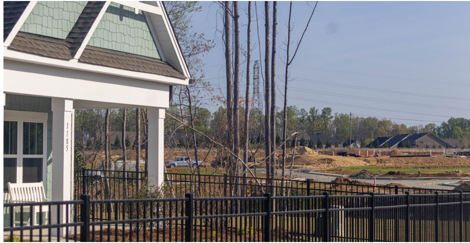
Housing development and construction on the PARC Northwest construction site April 2 on University Drive.
