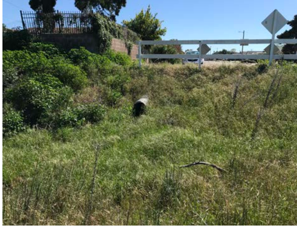
Photograph 2. View of a culvert that drains onto the subject property located along the eastern boundary, facing east.
