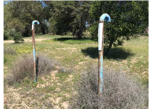
Photograph 6. View of two vent pipes located in the southwestern corner of the subject property.
