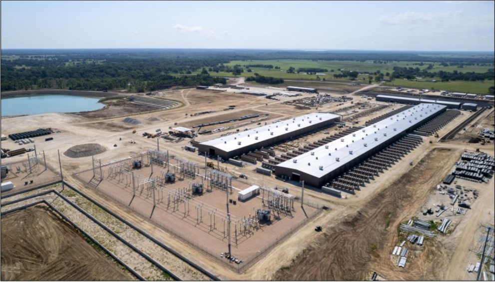
400 MW Substation at Corsicana Facility - Corsicana, Texas
