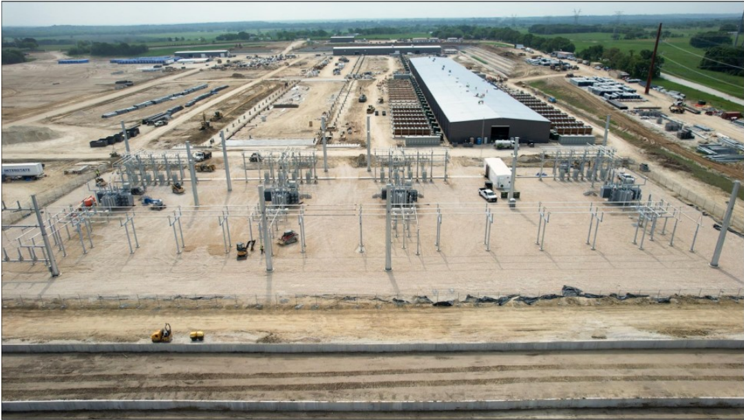
400 MW Substation at Corsicana Facility - Corsicana, Texas
