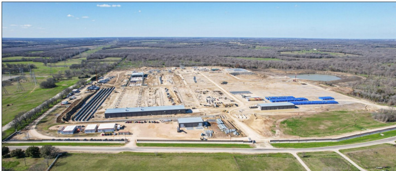
1 GW Corsicana Facility Development – Corsicana, Texas
