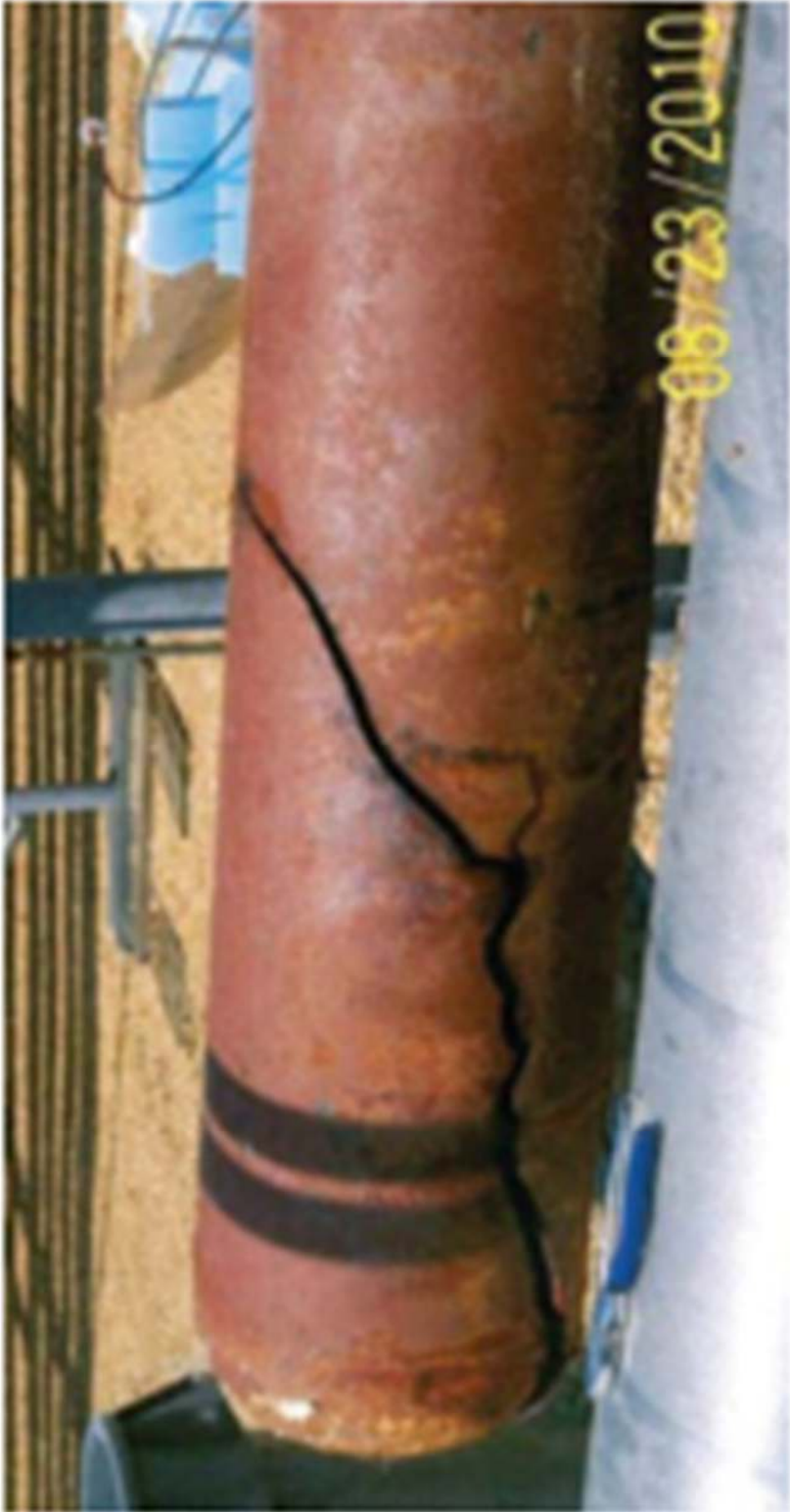
Figure 2. 12" LTRS line rupture; Millard - Mobile, AL (CSB Safety Bulletin #2010-13-A-AL, Jan 2015).
