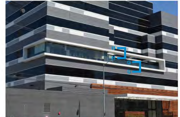
4TH LEVEL FRAMED ELEMENT HUNG FROM STRUCTURAL STEEL CURTAIN WALL ABOVE WAS SUPPORTED @ EACH INDIVIDUAL MULLION
