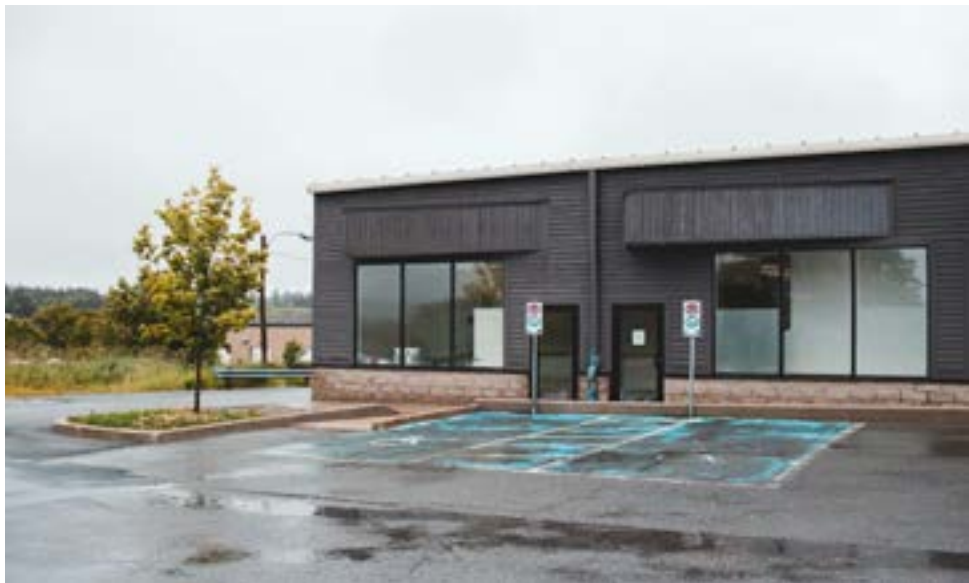
Image 2: Accessible route would require pedestrian travel behind parked vehicles into the drive aisle.
