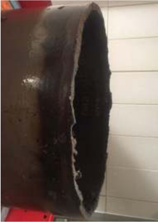
Figure 3. Pipe with end cap removed by hydraulic shock.
