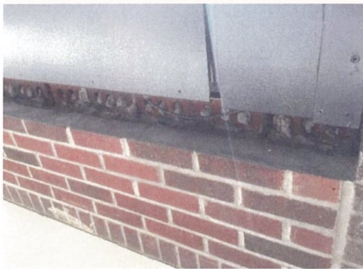
Figure 5: Below window wall missing brick course
