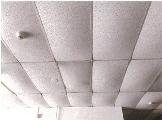
Figure 6: Typical sagging ceiling
