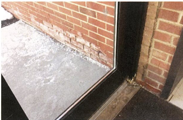
Figure 9: Efflorescence and C10 door
