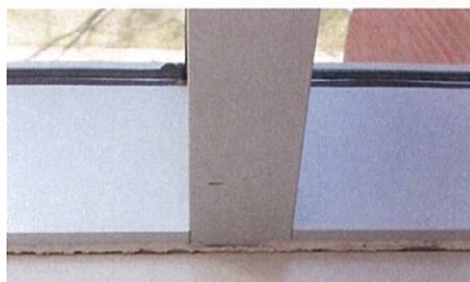
Figure 6: Window caulk cracking
