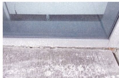
Figure 8: Deteriorating caulk at building base and sidewalk
