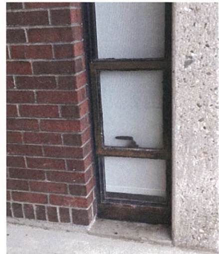
Figure 8: Original Window condition
