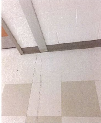
Figure 4: Cracked VCT where expansion joint is needed
