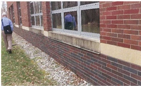
Figure 6: Window sill condition
