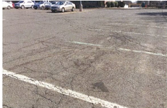
Figure 3: Typical parking lot cracks at front
