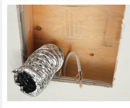
Existing 3" Duct and wiring
