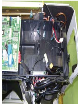
Replace New PCB
