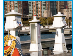
marine shore-power and dock lighting
