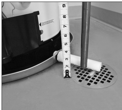
Figure 26 - Temperature and Pressure Relief Valve Pipe
